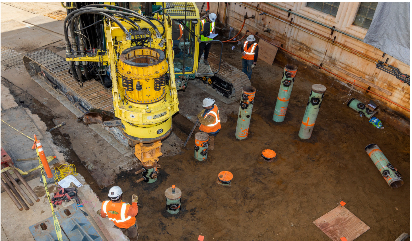
North Shore Pump Station Wet Weather Improvements: Driving 12 torque down piles into bedrock. The piles, along with rebar and concrete, will be part of creating a firm foundation upon which two ferrous chloride tanks will be placed.
