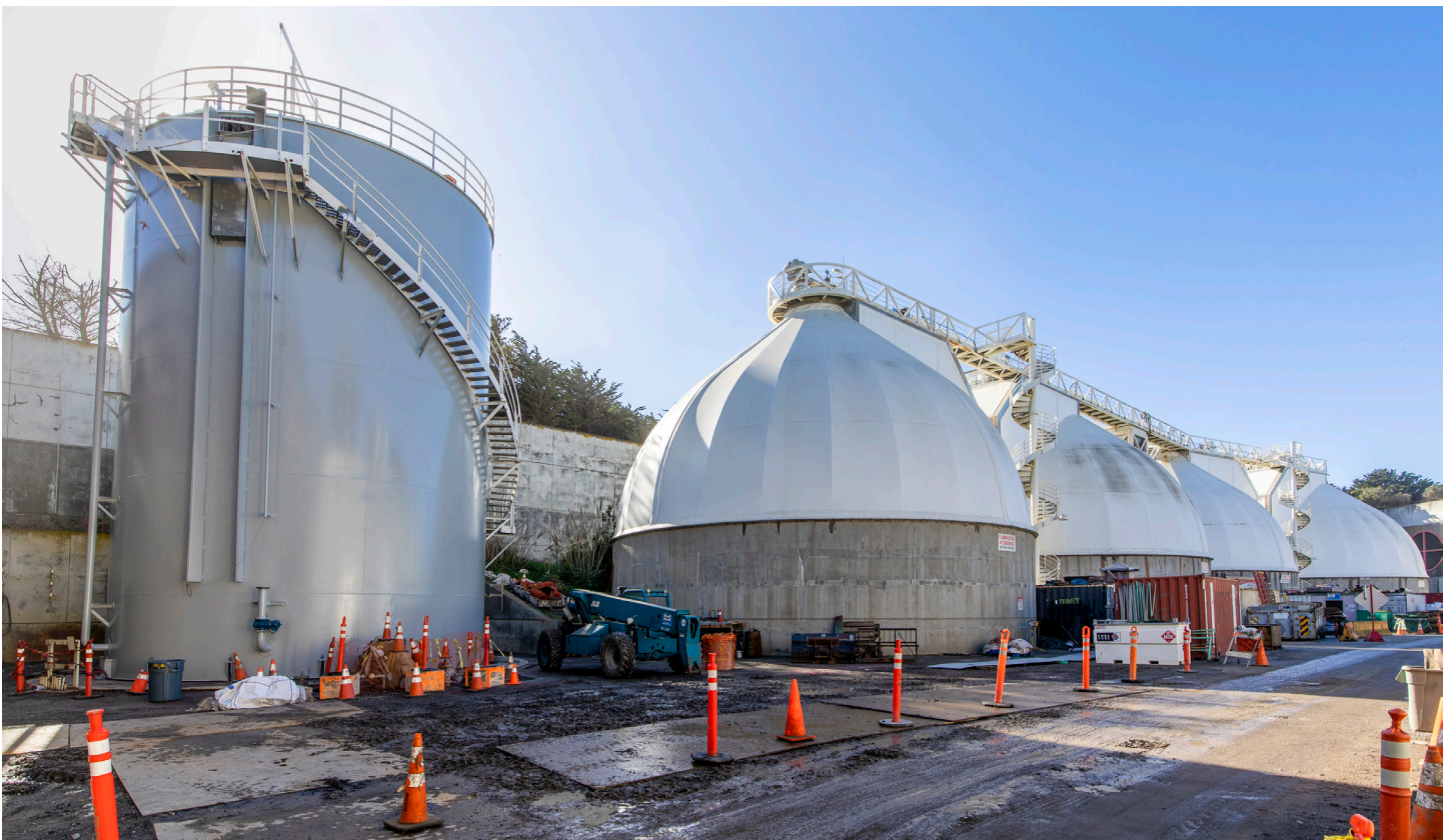
Oceanside Water Pollution Control Plant (OSP) Digester Gas Utilization Upgrade at left, the new biogas (methane) holder tank assembly (exterior coated grey, adjacent to existing egg-shaped digesters). On site Construction activities are on-going to include installation of new siloxane gas removal equipment, associated piping and onsite pavement restoration.
