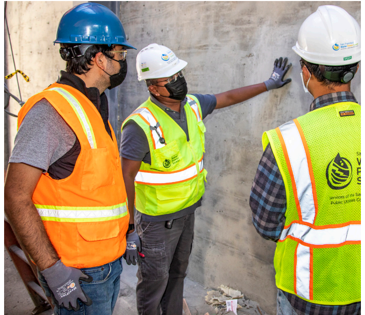
Project Engineer Alejandro Montero (BCI), Construction Management Bureau Lead Quality Assurance Inspector Arlando Victorio (Parsons) and Engineering Management Bureau Associate Engineer William Yu examining the concrete surface finish on the SEP Power Feed and Primary Switchgear Upgrades.
