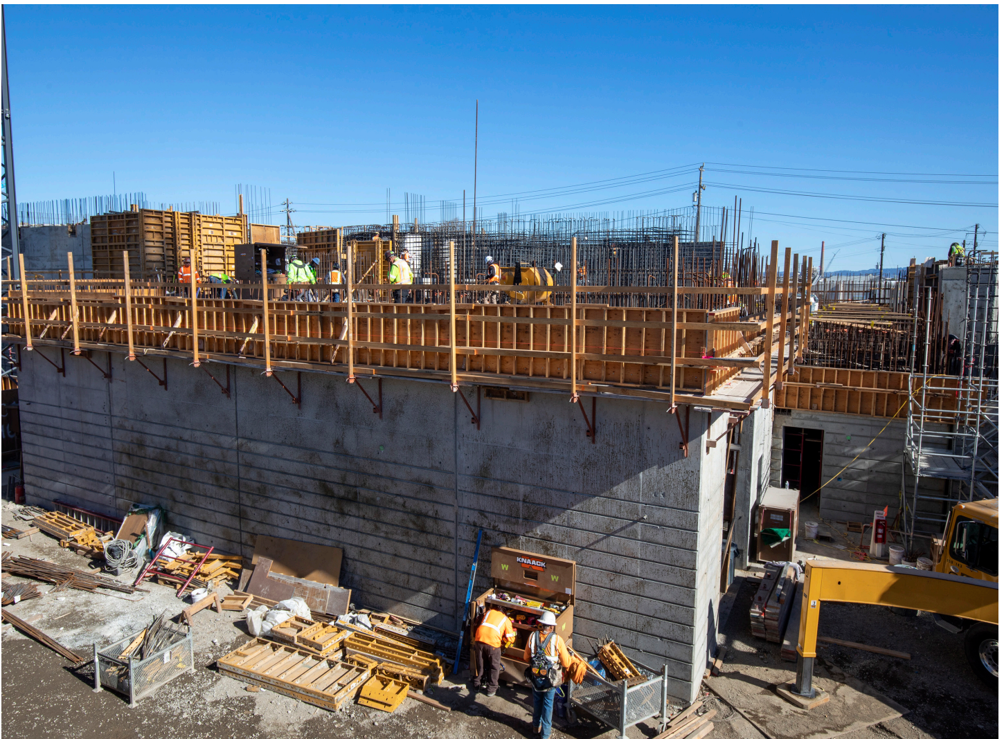
Crewmembers working on the Grit Tank Area at the new Headworks Facility Project at the Southeast Treatment Plant.
