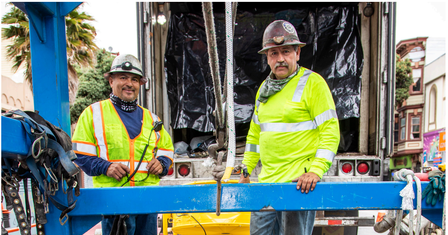
Crewmembers on the Mission Street, 16th to Cesar Chavez, Brick Sewer Rehabilitation Project. The project uses a trenchless method called cured-in-place pipe (CIPP) technology to rehabilitate the brick sewer tunnel. CIPP lining is pulled into place and cured with hot water.
