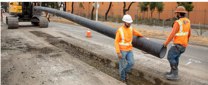
Cargo Way Box Sewer Odor Reduction Project: 14-inch HDPE (High Density Polyethylene) pipe being lowered into the trench. Pipe is being joined together by electro-fusion couplings.
