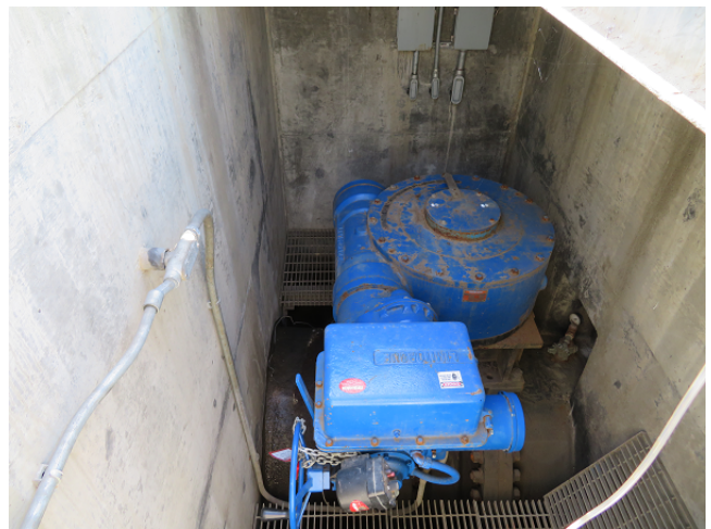
Typical Valve Vault
