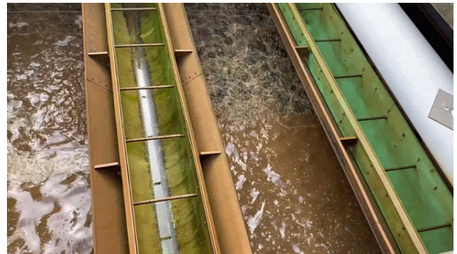
Inefficient Filter Media Backwashing
