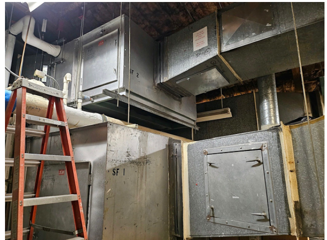
Existing Fans inside the Millbrae Yard Administration Building
