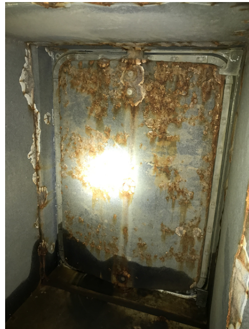
Corrosion on Existing Sludge Collection Auger
