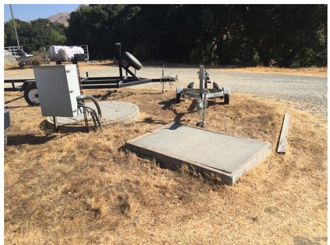
Existing Sewer Pump Station
