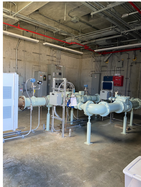
Typical Groundwater Station Piping
