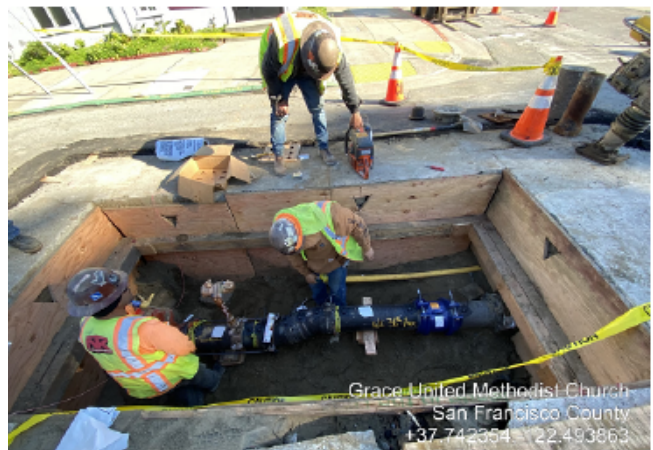
Installation of Cathodic Protection for 16-inch Steel Casing on 36th Avenue crossing Taraval Street for the L-Taraval Improvement Project
