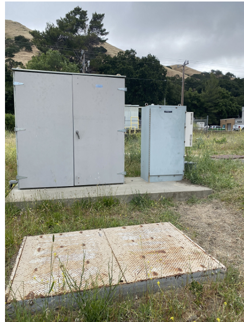
RIO Panel to be Upgraded
