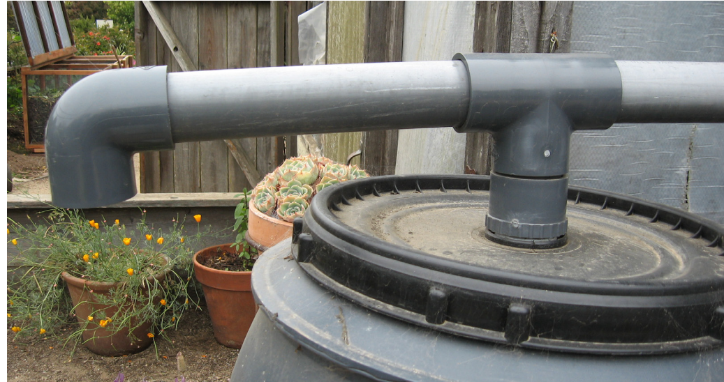
Overflow directed to an approved drain at Garden for the Environment
