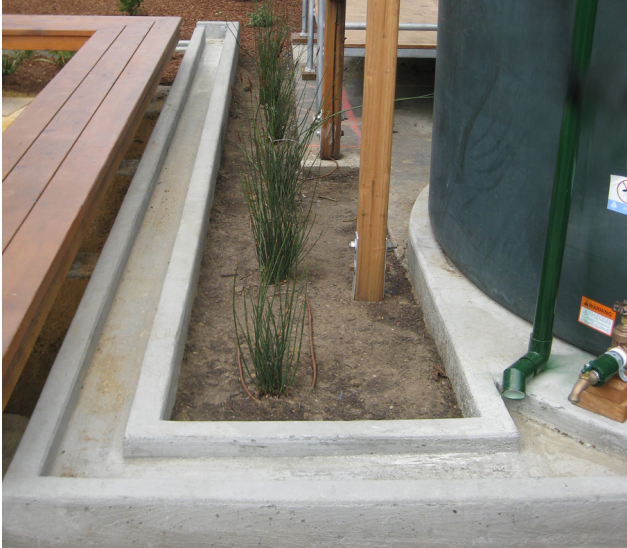
Overflow directed to a rain garden at Lafayette Elementary
