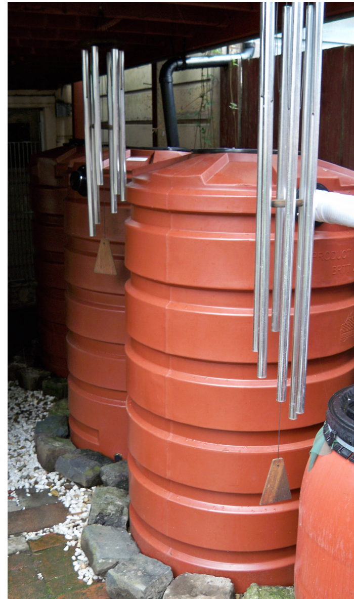
Rainwater harvesting system at a local residence
