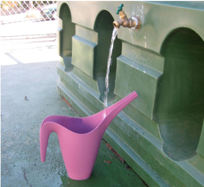
Filling a watering can with a hose bib
