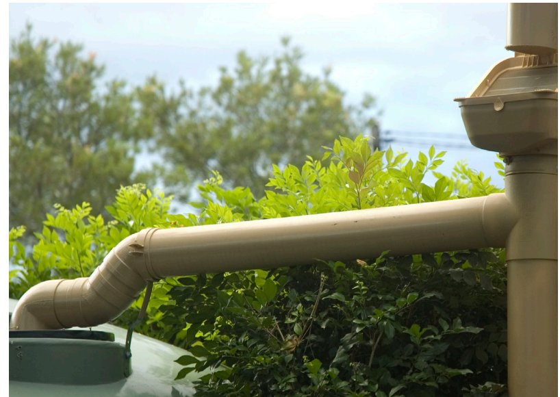
Downspout connection with debris excluder
