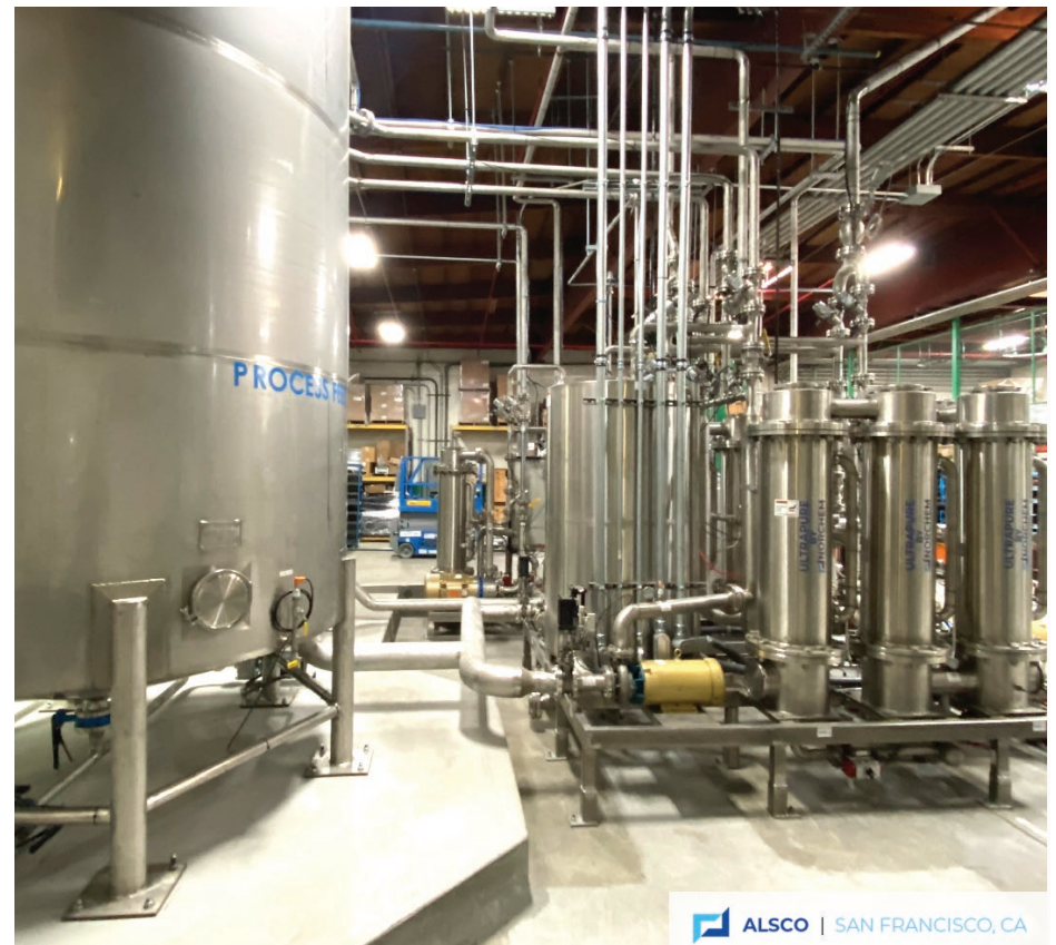
Ultra-Pure Water Process Equipment at ALSCO
