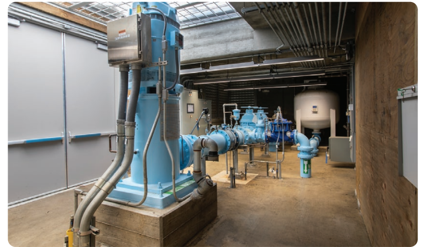
Golden Gate Park Central groundwater well station site
