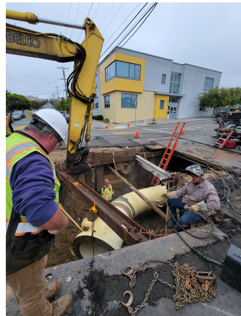
Welding the straps on 36 welded steel pipe for Potable Emergency Water for Firefighting on Vicente Street
