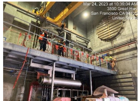
OSP Building 800 new cogeneration engine room steel mezzanine construction, installation of co-gen engine combustion exhaust system rough-in in March 2023
