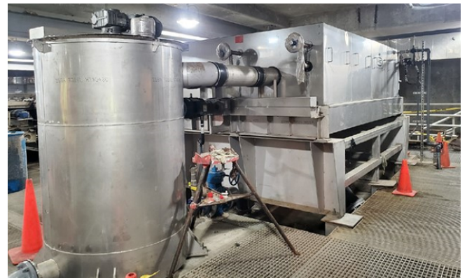
Proposed new Rotary Drum Thickener (RDT) and associated flocculation tank assembly
