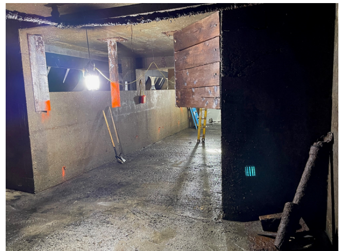
Baker St. CSD Damaged Baffle Wall
