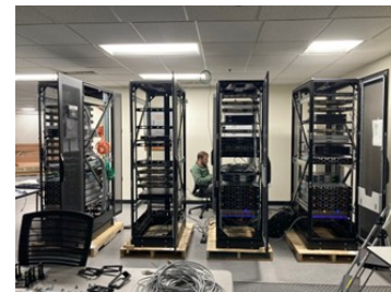
Southeast Water Pollution Control Plant DCS Hardware Operation Readiness Test (ORT)
