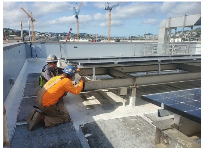
Photovoltaic (PV) System on Roof of SEP 032
