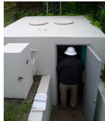
Seacliff Pump Station No.1
