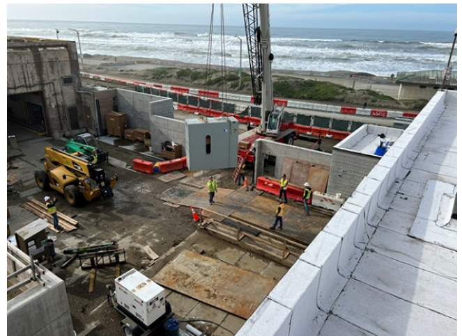
New electrical switchgear delivered to New Electrical Building in January 2023
