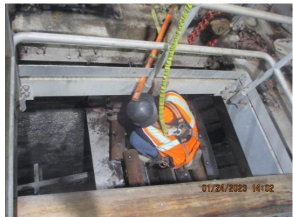
(E) WW-648 OSP Building 042 Primary Clarifier Improvements: □ Contractor performing selective demolition of existing helical scum skimmer assembly within Clarifier Tank No. 1
