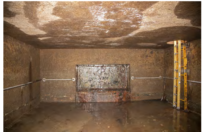
Brannan CSD Existing Damaged Butterfly Discharge Valve
