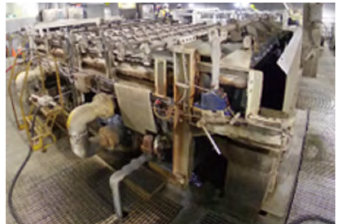
Existing Gravity Belt Thickener identified for equipment replacement.
