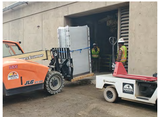
New Distributed Control System (DCS) cabinet delivery at a Southeast Water Pollution Control Plant (SEP) process building.
