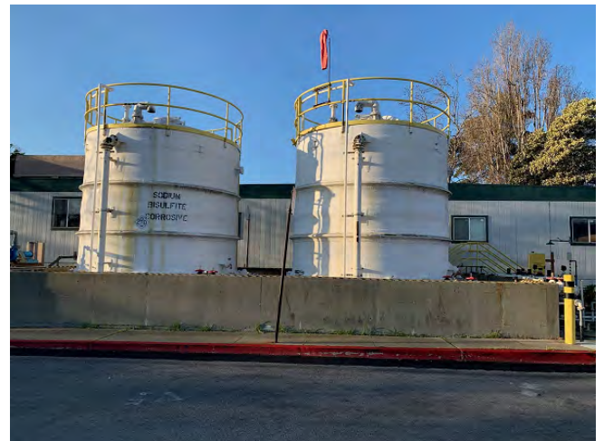
Existing Sodium Bisulfite Tanks
