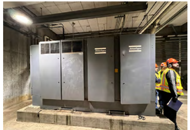
Existing pressure swing absorption compressor assembly equipment identified for replacement.
