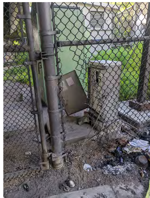
Security Issues at Cesar Chavez Pump Station
