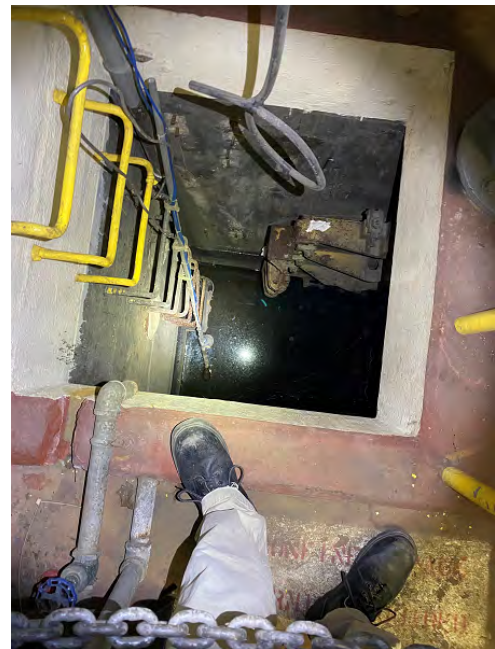
Wet Well of Pump Station
