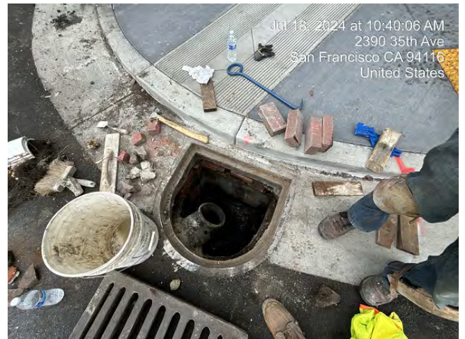
Segment B: Installing Catch Basin Sand Trap and Grouting Joints NE 35th Ave
