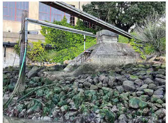
Damaged Rip-Rap Under and Around Laguna CSD
