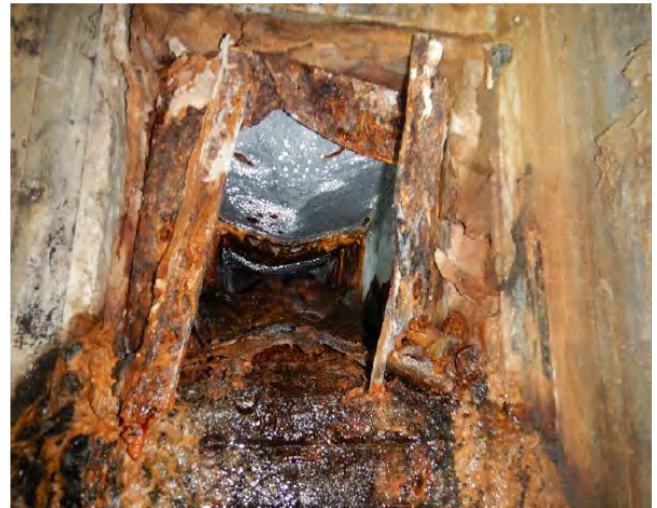
HVAC Ducting Corrosion Due to Water Intrusion
