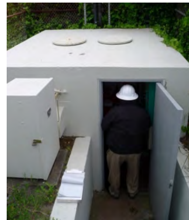
Seaclyff Pump Station No.1
