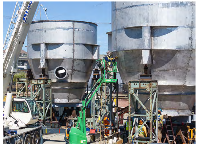
Welding on one of four Biosolids Storage Silos, which will be set in the Biosolids Dewatering Building.
