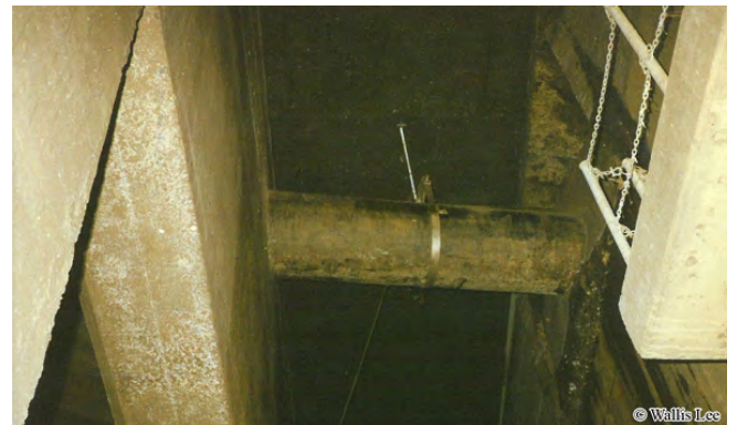
Existing Weir Structure where Marin Street Sewer Crosses over the Islais Creek Transport Storage Box
