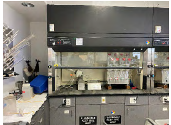
Existing fume hood #3 identified for replacement.
