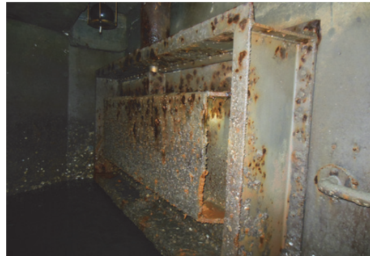
Non-operational butterfly valve at Brannan CSD
