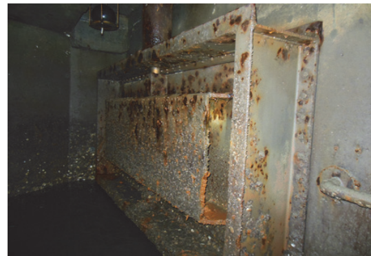
Non-operational butterfly valve at Brannan CSD
