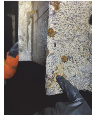
Corroded Baffle support at Baker Street CSD
