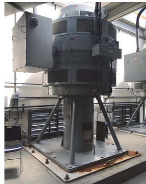
Main Pump Being Evaluated
