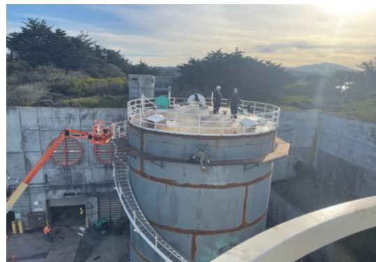
As of September 2021, the Contractor prepared a temporary enclosure on site, surface prepared and coated the new 741 digester gas holder roof assembly.
