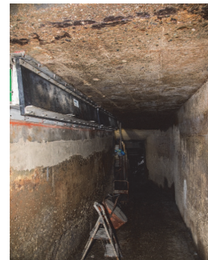
Inspection of walls/ceiling inside Jackson Sewer after shotcrete and the backflow valve installation
