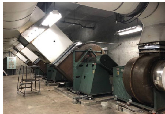
OSP Building 011 as-found condition of ventilation exhaust systems
