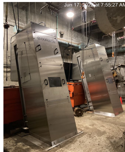
Completed bar screens in operation
