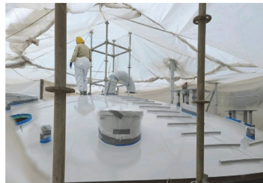
As of September 2021, the Contractor prepared a temporary enclosure on site, surface prepared and coated the new 741 digester gas holder roof assembly.
