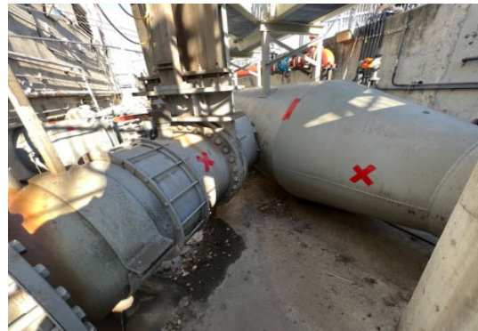
Locations of condition assessment areas identified by specialty consultant at discharge manifold.
