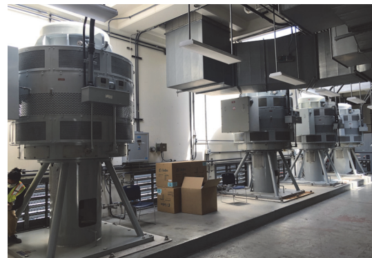
Pumps at SEP 550
