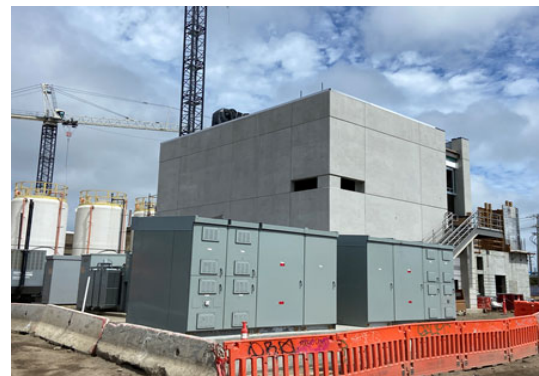
New Outdoor Metering Cabinets
