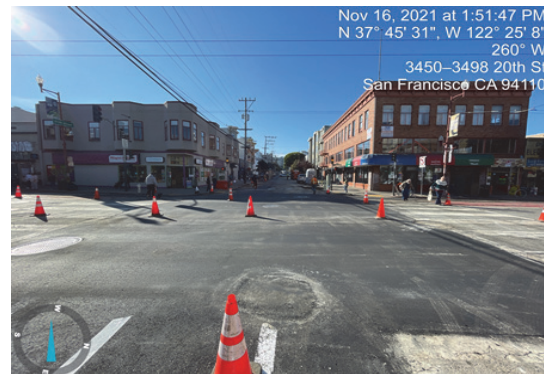
Paving at intersection of 20th and Mission completed after EFWS relocation work
