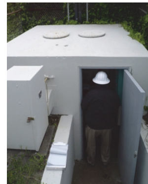
Seacliff Pump Station No.1
