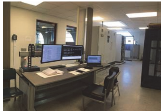
Updated Bruce Flynn Pump Station Control Room
