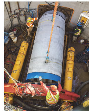
Microtunneling at jacking pit on Vicente Street between 19th and 20th Avenues. Lowering pipe segment--into the shaft.
