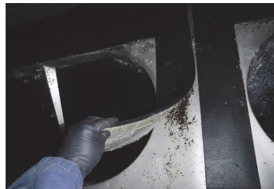
Baker St. CSD damaged backflow preventer valve
