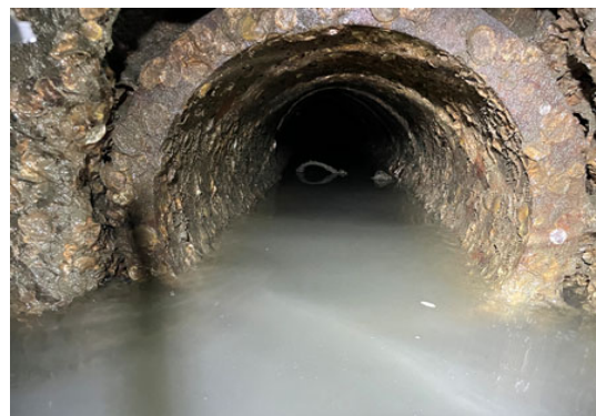
Howard St. CSD discharge pipe
