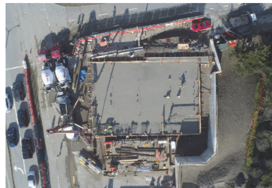
Drone Ariel Photo of New Electrical Building – Cast-In-Place Concrete Slab pour (January 2022)
