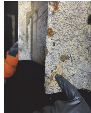
Corroded Baffle support at Baker Street CSD
