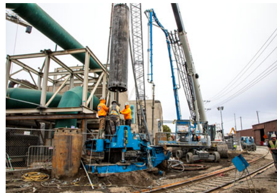
Drill Pier work for Pipe Rack in vicinity of Union Pacific Railroad Right-of-Way
