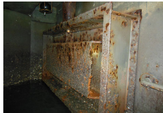
Non-operational butterfly valve at Brannan CSD
