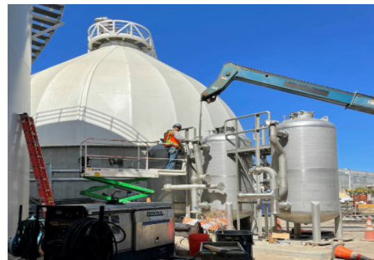
Contractor installing the new stainless steel digester gas siloxane removal system as of May 2022.
