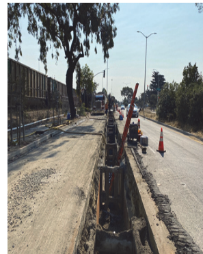
Excavation and laying HDPE flush line pipe at Cargo and Mandel St
