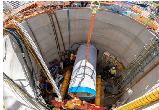
Contractor is installing the final pieces of the sewer tunnel through the launching shaft at 20th Ave and Vicente St.
