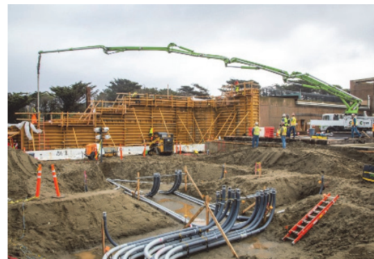
Placement of concrete for the East retaining wall on site in November 2021
