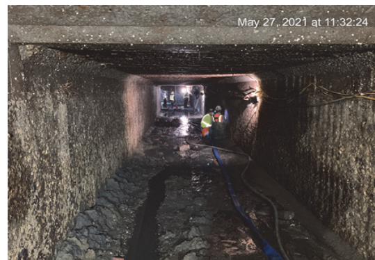
Concrete crack survey in Jackson Street CSD
