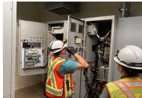
North Shore Site Visit: Dry Weather Pump Variable Frequency Drive (VFD)
