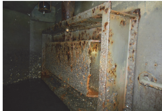
Non-operational butterfly valve at Brannan CSD
