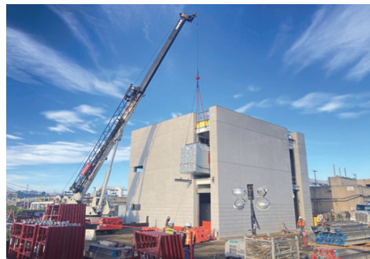
New switchgear being installed on the second floor of the new Primary Switchgear Building SEP 032
