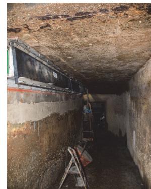
Inspection of walls/ceiling inside Jackson Sewer after shotcrete and the backflow valve installation
