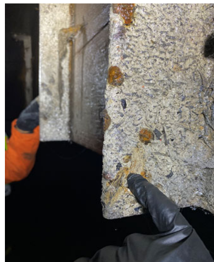
Corroded Baffle support at Baker Street CSD
