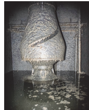
Pump 3, suction pipe
