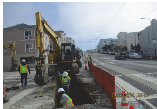
Contractor excavating sewer trench line from north manhole downstream to the existing manhole at the intersection of 34th Ave and Taraval Street.
