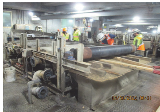
Selective equipment demolition to GBT No. 1; this work is expected to be completed prior to the project contract work commencing on the replacement of GBT No. 2 and GBT No. 3.
