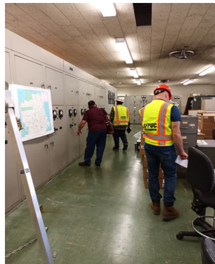
WWE staff and design team surveying existing obsolete electrical equipment at NPF 930 Administration Building.
