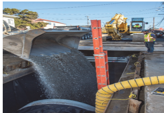
Preparing to install 54-inch reinforced concrete sewer pipe on Vicente Street between 33rd and 34th
