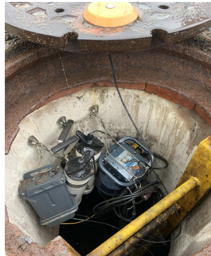
Existing field instrumentation equipment installed in a sewer manhole
