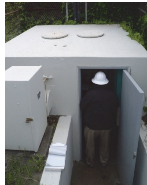
Seacliff Pump Station No.1
