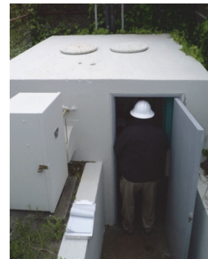
Seacliff Pump Station No.1
