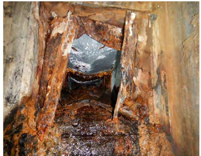
HVAC Ducting Corrosion Due to Water Intrusion
