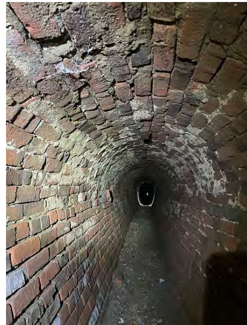
Investigation of 3ft x 5ft Brick Sewer on Folsom Street as Part of Contract WW-719A
