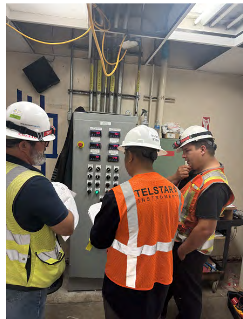
Main Gates Panel Startup and Testing
