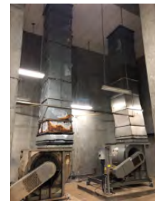
Building 200 Supply Fans with Corroded and Deficient Ductwork Identified for Replacement
