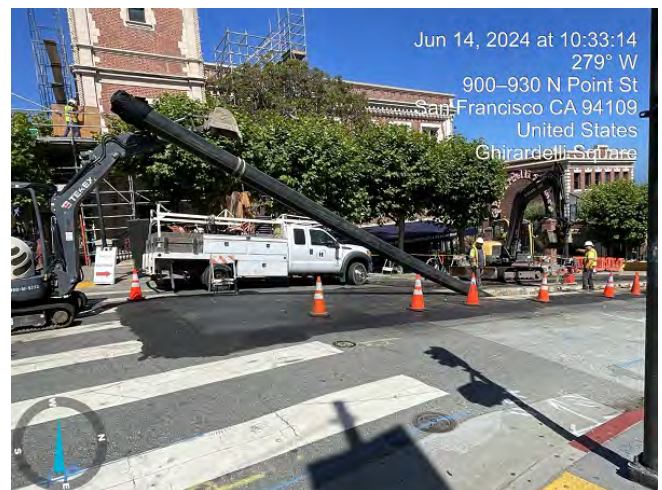
Backfilling an Open Excavation Trench After Replacement Installation of a 12-inch Main Sewer on Phelps Street, San Francisco
