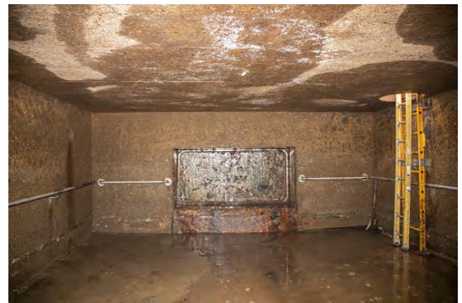
Brannan CSD Existing Damaged Butterfly Discharge Valve
