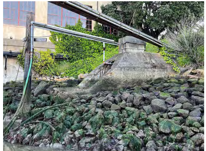
Damaged Rip-Rap Under and Around Laguna CSD
