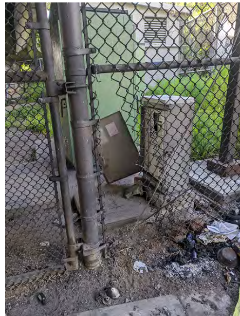
Security Issues at Cesar Chavez Pump Station
