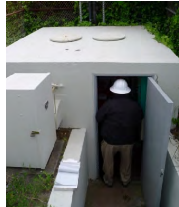
Seacliff Pump Station No.1
