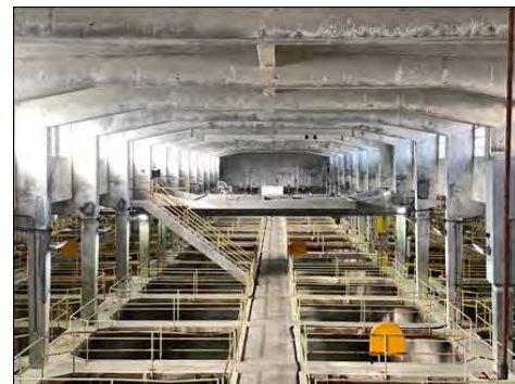
NPF 041 Main Sedimentation Tank Area
