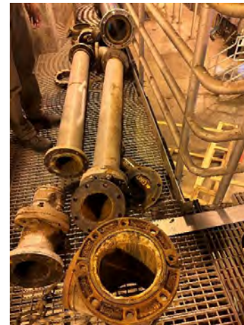
WW-669 contract, within Building 011, the Contractor continues selective Hydrogritter Pipe Demolition and Removal
