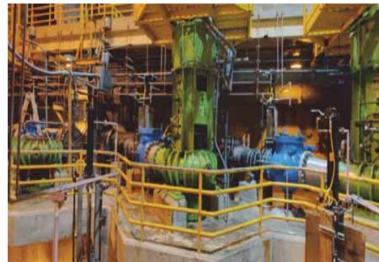
Existing Dry Weather (DW) Pump
