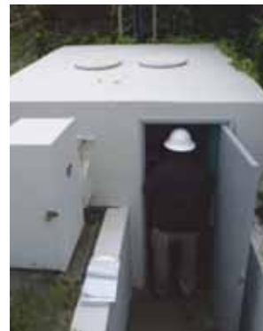
Seacliff Pump Station No. 1
