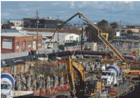
Underslab earthwork and concrete activities at primary influent distribution area and grit tank/handling area.
