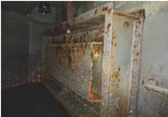
Non-operational butterfly valve at Brannan CSD
