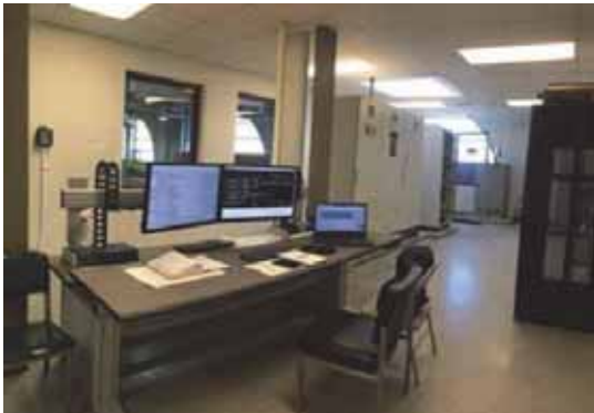
Updated Bruce Flynn Pump Station Control Room
