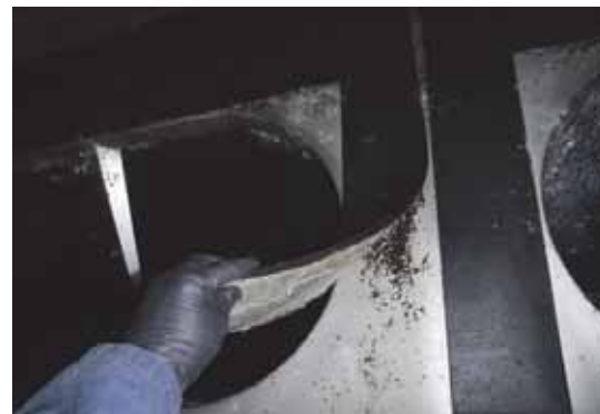
Baker St. CSD damaged backflow preventer valve
