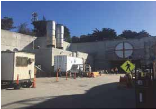
The trailer-mounted temporary boiler (white) installed at the base of flare building 821 has been on-line in March 2021.
