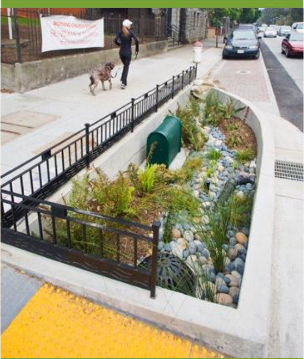
INNOVATIVE STORMWATER MANAGEMENT SOLUTIONS
