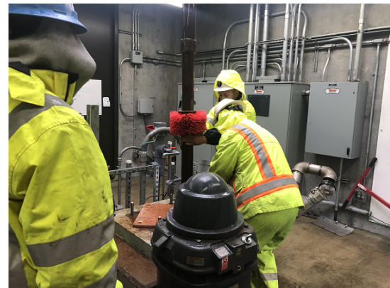
Well brushing at Colma BART Well Facility as part of Phase 2A (Contract C) WD-2878A
