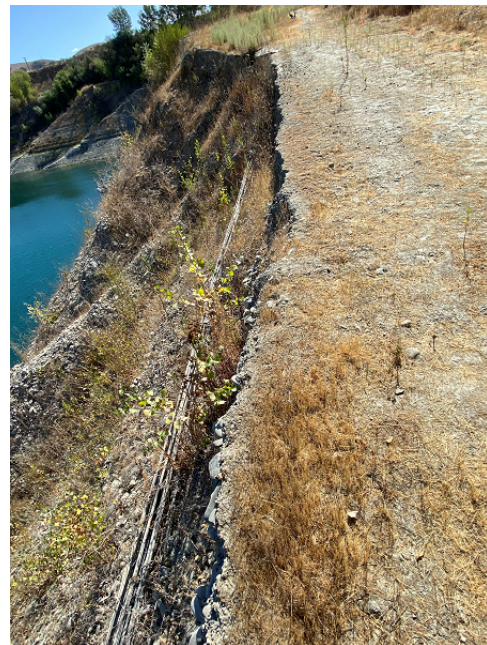
Erosion Along Access Road
