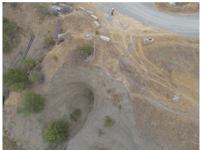
Pond F2 Bank Erosion Area
