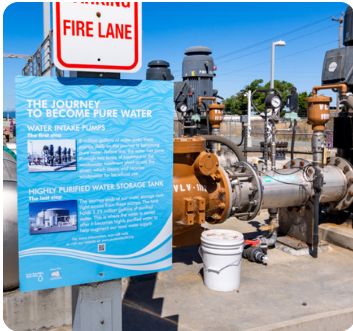
Silicon Valley Advanced Water Purification Center, San Jose, CA
