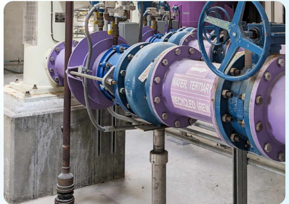
Inside the Westside Recycled Water Treatment Facility
