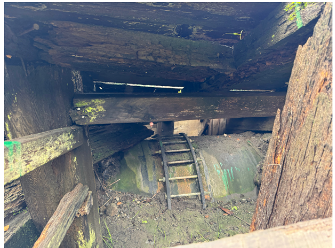
Flexible Joint Coupling and Housing to be Upgraded
