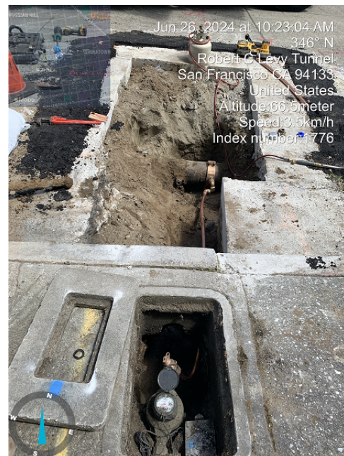
Galvanized Steel Water Service Pipe, with Lead Whip, replaced with Copper Piping
