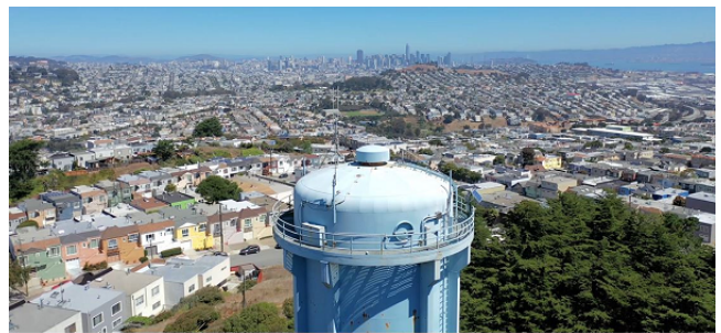
Exterior Drone Photos Taken Following Testing and Inspection of Tank Interior and Exterior Coatings at La Grande Tank
