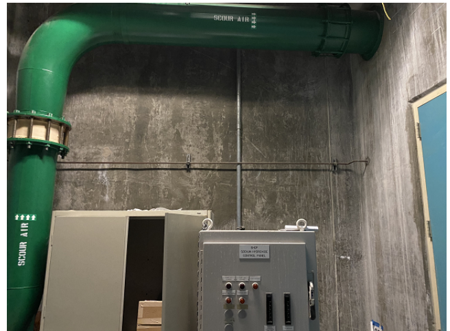
Air Scour Blower Room at the Harry Tracy Water Treatment Plant
