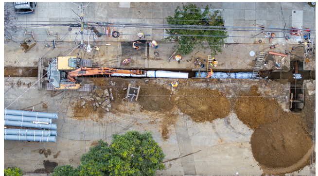
Installation of Earthquake Resistance Ductile Iron Pipe for the Hampshire Street Project
