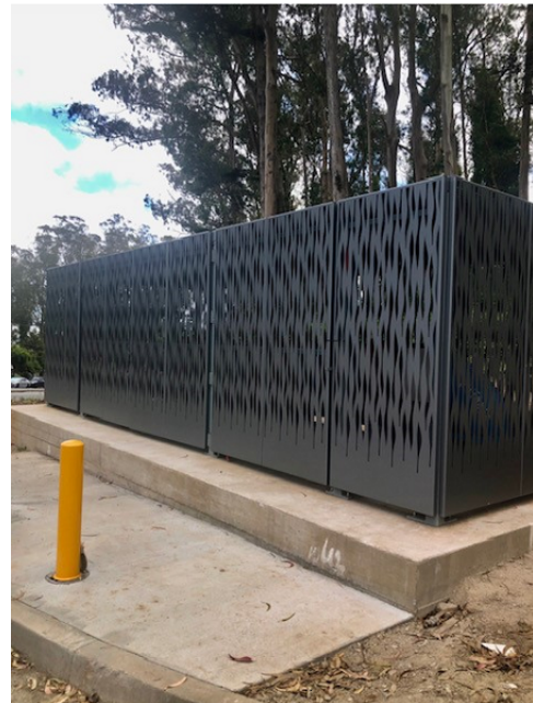
Enclosure Installation for Clarendon Supply Facility at Dellbrook and Clarendon
