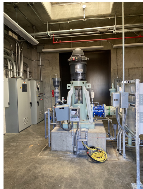
Typical Groundwater Station Equipment
