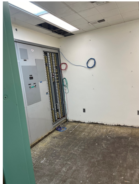
Main Control Panel to be Removed
