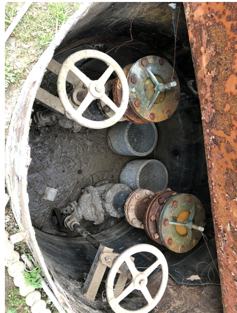
Air Valves to be Upgraded
