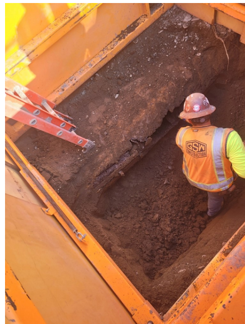
Existing 30-inch Pleasanton Pipeline Break along Spring Line
