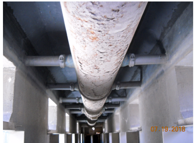
Corrosion on Existing Air Scour Pipeline at the Sunol Valley Water Treatment Plant
