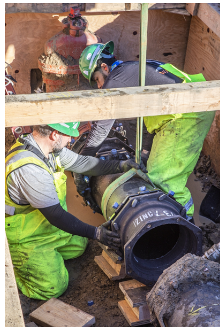
CDD Crews performing a water main connection on newly installed ductile iron pipe on Contract WD-2843 (Diamond Street).
