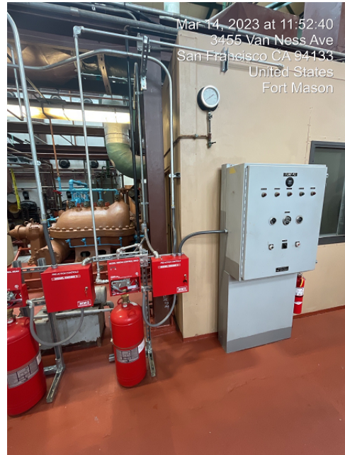
EFWS Pump Station No. 2
