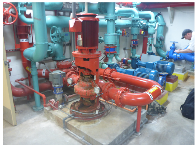
Existing Fire and Utility Water Pumps
