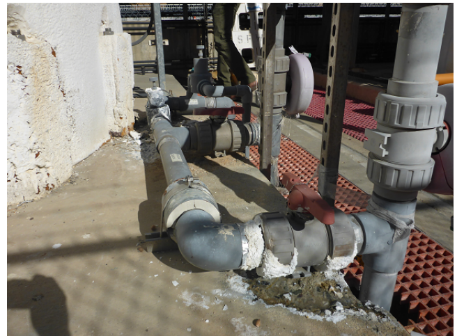
Concrete Damage at Caustic Soda Line
