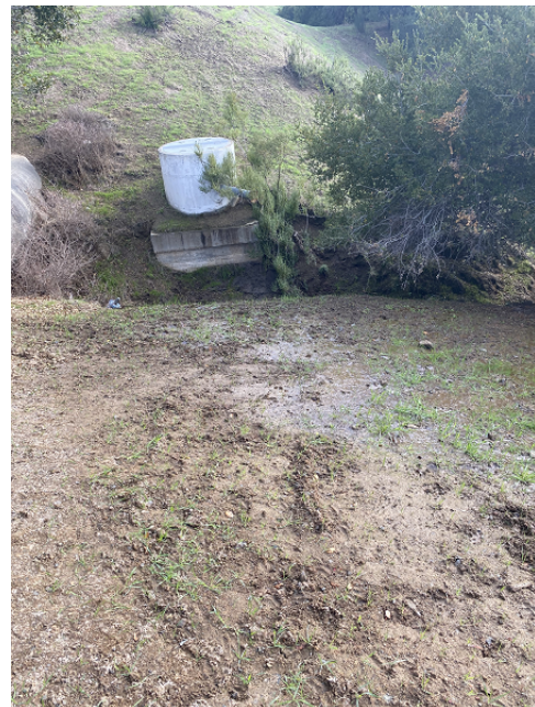
Segment of Pipeline on Hilly Terrain with an Active Leak
