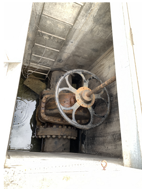
Valve Requiring Installation of an Additional Valve for Safe Pipeline Entry
