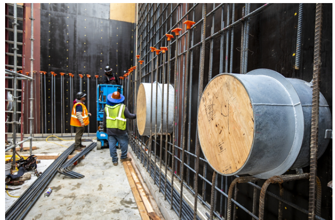
Installation of 24-inch diameter Earthquake Resistant Ductile Iron Pipe reservoir inlet pipe
