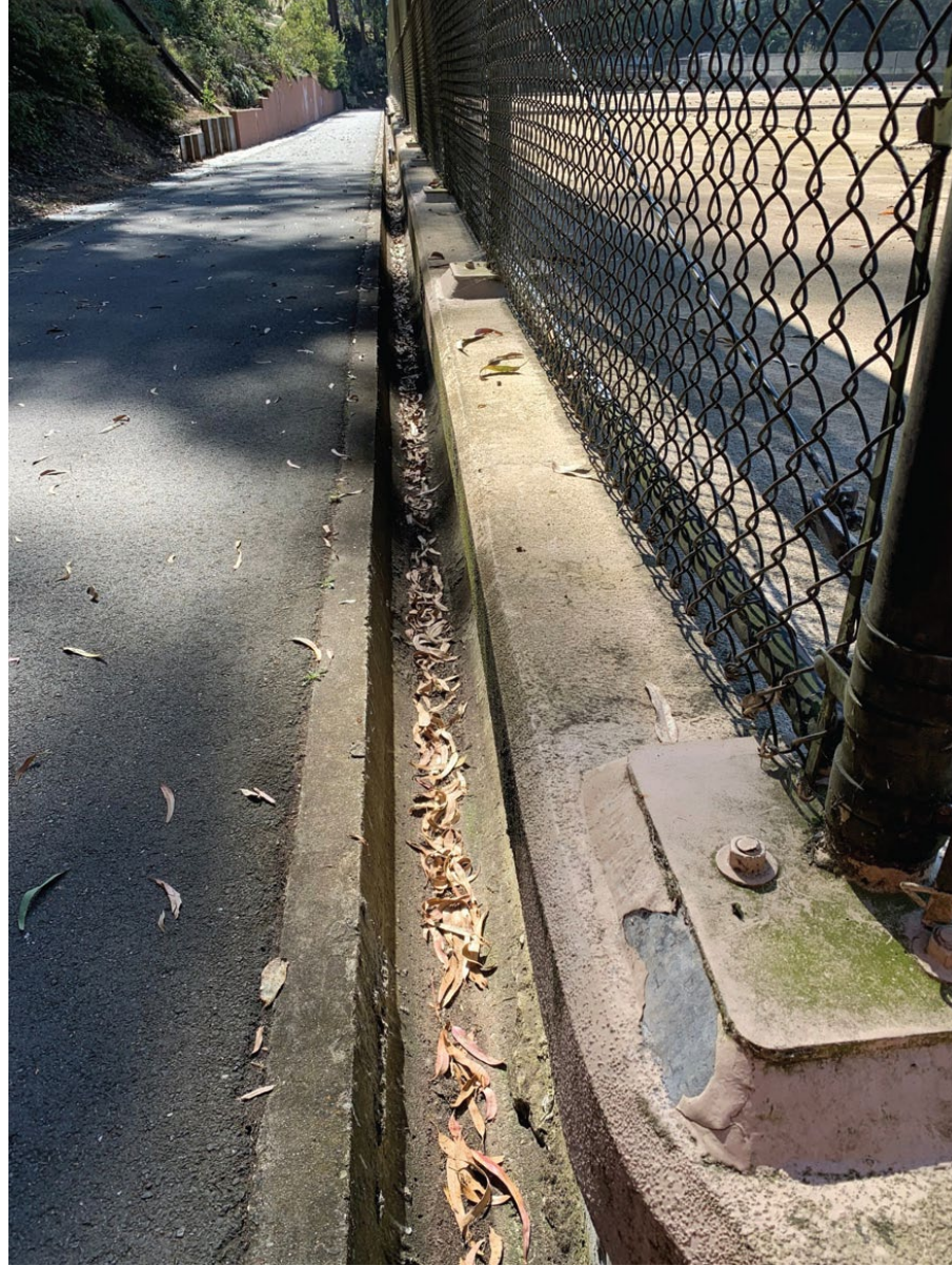
This concrete channel wall nearest the asphalt pathway at Sutro Reservoir will be raised to enhance safety for people and their pets.
