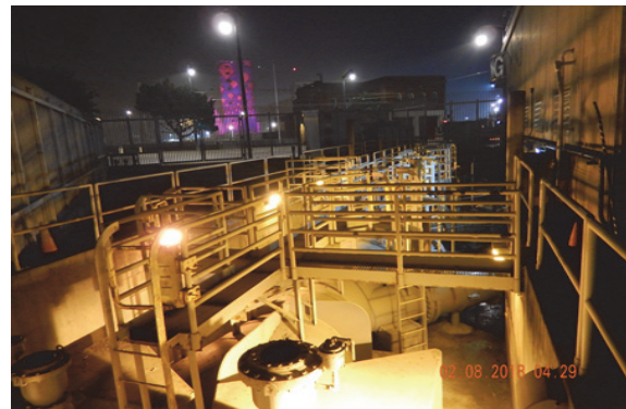
Booster pump manifold pit illuminated before sunrise
