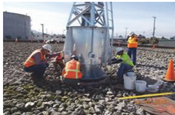
At the Existing Wastewater Treatment Plant, installation of a new rock trickle filter rotary distributor arm was completed in the Summer of 2016.
