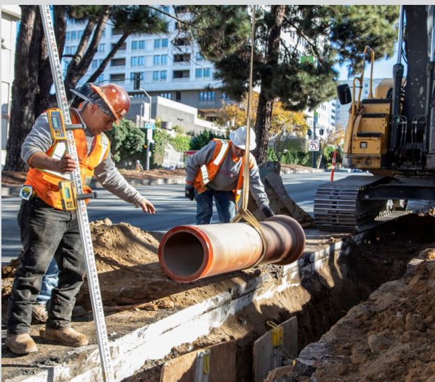
Geary Boulevard Water Main Installation and Sewer Replacement Project (Segment B): Replacing and repairing aging sewer mains.
