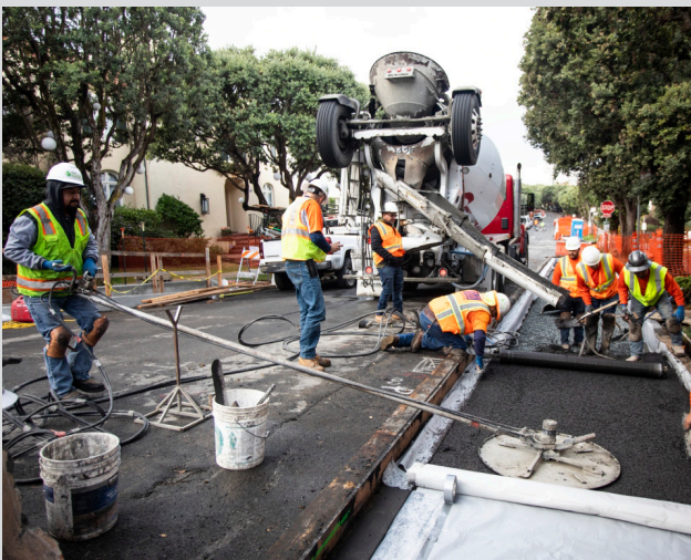
Baker Beach Green Streets Project: Sea Cliff Avenue 25th Street Avenue to 26th Avenue. Pervious concrete installation: A special type of porous concrete that allows stormwater to pass through and soak into the ground in contrast to hard surfaces such as asphalt or traditional concrete where stormwater runoff flows into the sewer system.
