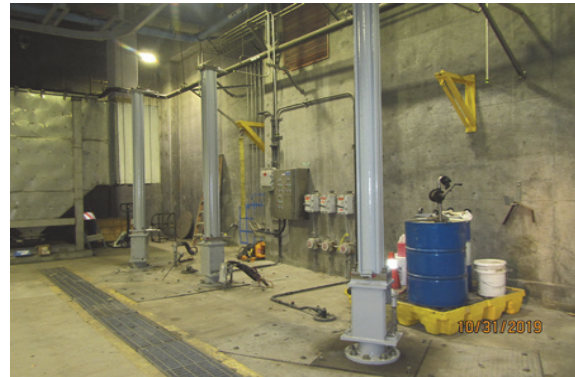
HPU cylinders showing new sluice gates
