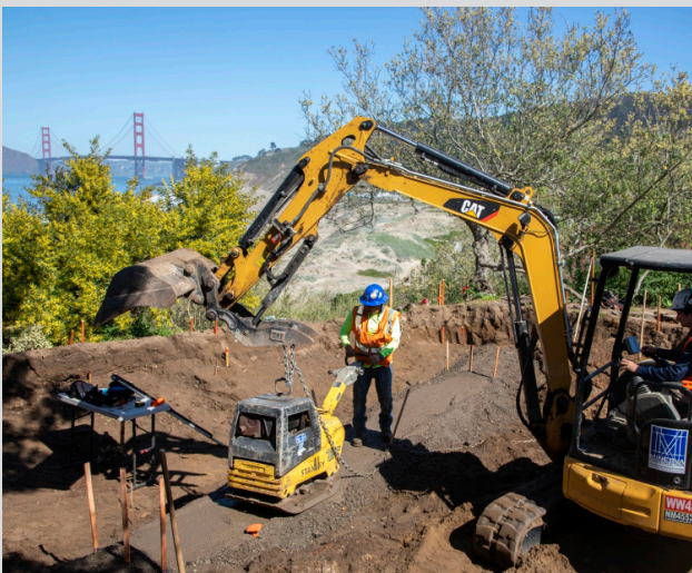
Baker Beach Green Streets Project: New rain gardens at California Coastal Trail access entrance at 25th Avenue to Baker Beach. Excavation.
