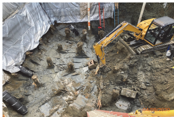
Excavation for new pump station and exposing existing timber piles from demolished pump station
