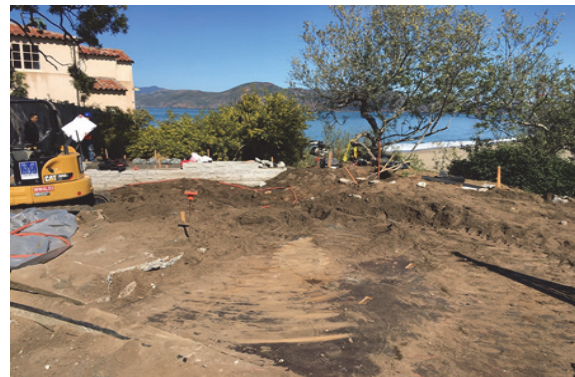
View of rain garden construction at 25th Ave North within Golden Gate National Recreation Area
