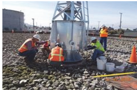
At the Existing Wastewater Treatment Plant, installation of a new rock trickle filter rotary distributor arm was completed in the Summer of 2016.
