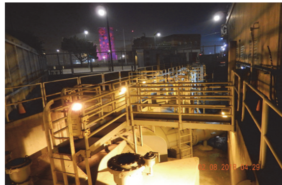
Booster pump manifold pit illuminated before sunrise
