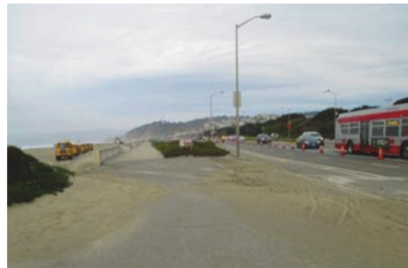
Contractor excavator and dump trucks loaded with surplus sand collected at North Ocean Beach
