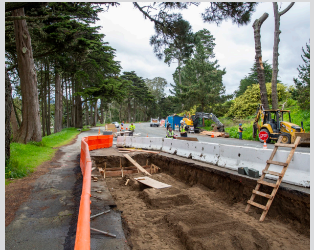
Baker Beach Green Streets Crews construct the subsurface infiltration gallery trenches across the roadway (an underground stormwater storage structure filled with gravel that receives runoff through horizontal pipes below the pavement surface)
