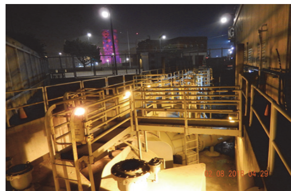
Booster pump manifold pit illuminated before sunrise
