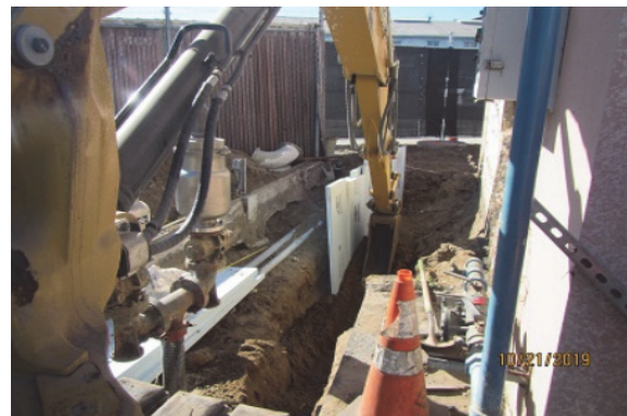
Insulation for Relocated Dewatering Line
