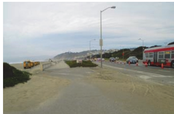
Contractor excavator and dump trucks loaded with surplus sand collected at North Ocean Beach
