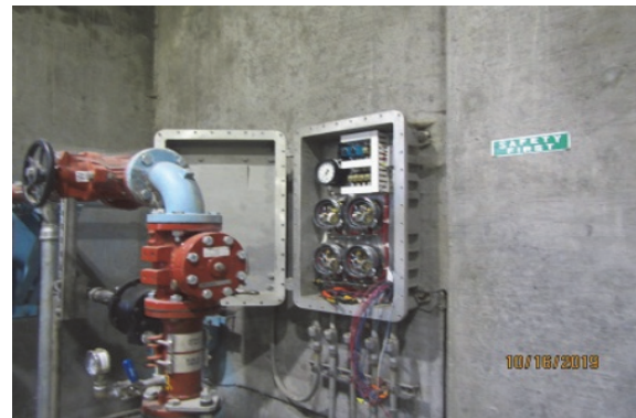
New W2 Pump Control Panel
