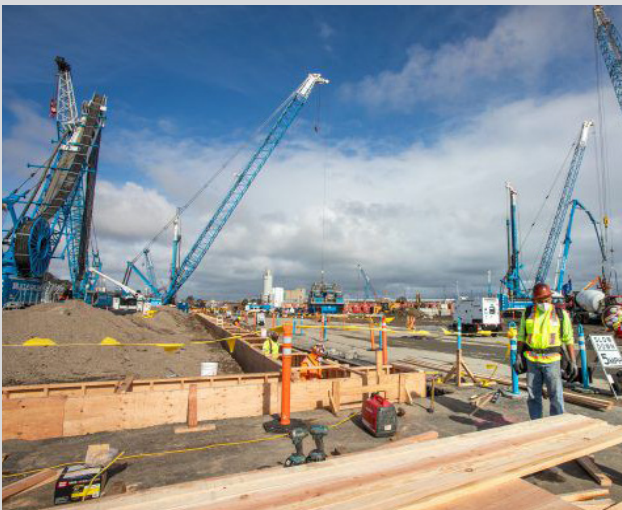
Southeast Wastewater Treatment Plant: Construction of a starter wall for the slurry wall 150-ft down to cut off groundwater. Site where digesters will be placed.
