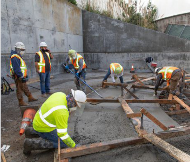
Oceanside Treatment Plant: Digester Gas Utilization Upgrade Project - Concrete pour on future location of gas holder tank that will hold excess digester gas that does not get used up.
