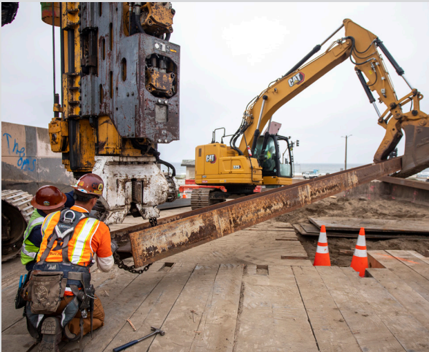
Westside Pump Station Reliability Improvements: Drilling & Shoring 50-feet and 2-inch steel pier.
