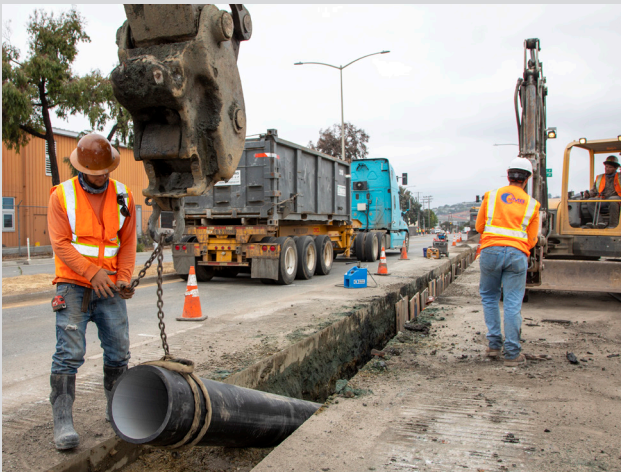
Cargo Way Box Sewer Odor Reduction Project: 14-inch HDPE (High Density Polyethylene) pipe being lowered into the trench. Pipe is being joined together by electrofusion couplings. Contractor is excavating for one pipe at a time and then pipe is installed due to the bad ground conditions.
