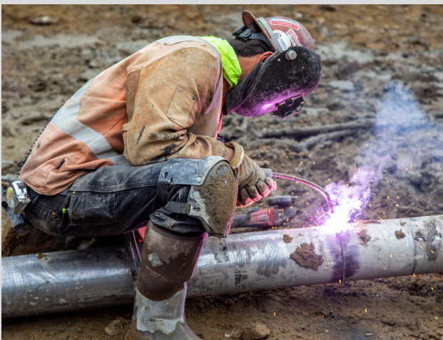
Southeast Wastewater Treatment Plant: Biosolids Digester Facilities Project: Perry Savas, Malcolm Drilling welder.
