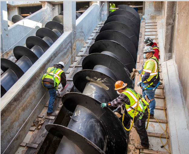
Southeast Water Pollution Control Plant Buildings Mechanical Improvements: Auger Screw Pumps Install in SEP Building 062, Screw Pumps 1, 2, 3: Grout Screw Pump Troughs. Grout Screw Pump No. 3.
