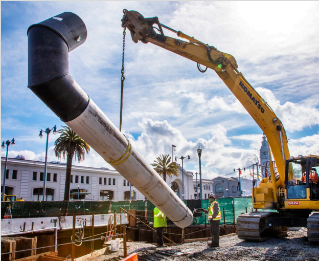
Force Main Rehabilitation at Embarcadero and Jackson Improvements (FMEJ): Lowering 28-inch pipe, slip lining in Pit 3, under the Embarcadero going towards Pit 2.
