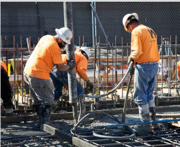
Mariposa Pump Station Improvements Project: Concrete pour for first floor of pump station.
