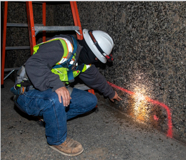
Southeast Wastewater Treatment Plant: Channel in Building 540 for effluent discharge to the booster station at Islais Creek. Superintendent, Bay Engineering, LLC, Matt Cox, examines cracks in the concrete that need grouting before the coating is applied.
