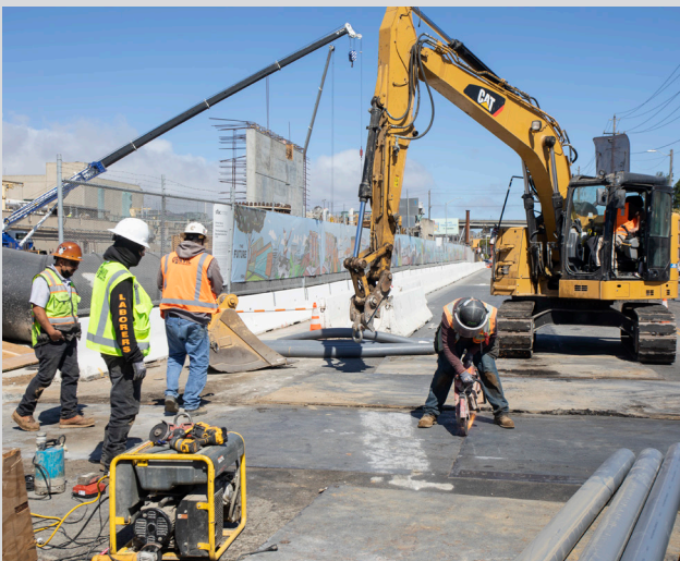
Bay Corridor Transmission and Distribution Phase 2 DB-129.2: Tie-in for duct bank from existing substation to new Bay Corridor Substation DB-130. This work includes placing conduits and trench cards in trench at Evans Avenue and Quint Street (Southeast Wastewater Treatment Plant [SEP]). Work will continue on Quint Street and then Davidson Avenue.
