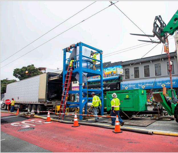
Mission Street, 16th to Cesar Chavez, Brick Sewer Rehabilitation Project: The project uses a trenchless method called cured-in-place pipe (CIPP) technology to rehabilitate the brick sewer tunnel. CIPP lining is pulled into place with water and cured with hot water.
