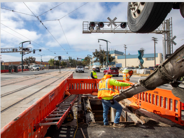
Cargo Way Box Sewer Odor Reduction Project: Concrete pour on southbound lane of Third Street at Cargo Way for the base of the manhole. Concrete elephant trunk method of pouring concrete.
