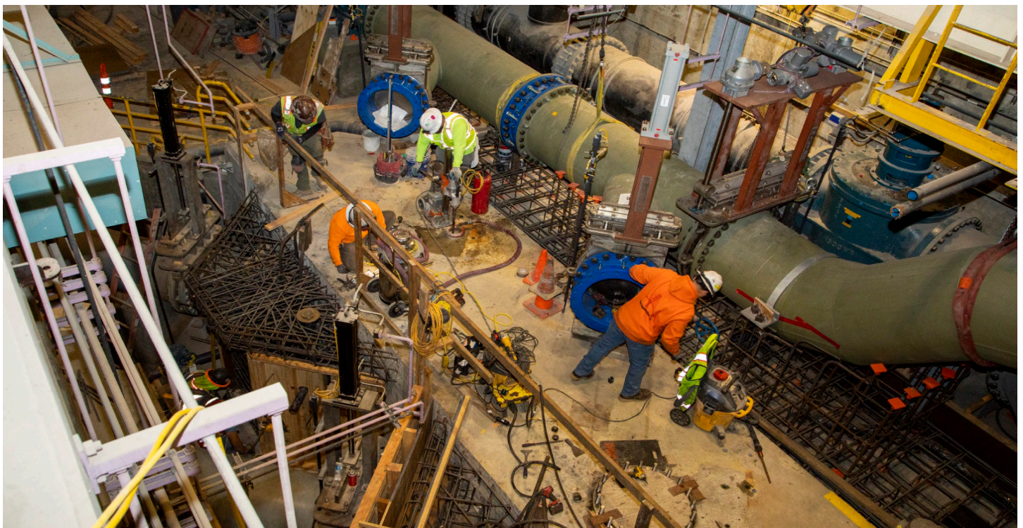
North Shore Pump Station Wet Weather Improvements: Driving 12 torque down piles into bedrock. The piles, along with rebar and concrete, will be part of creating a firm foundation upon which two ferrous chloride tanks will be placed.
