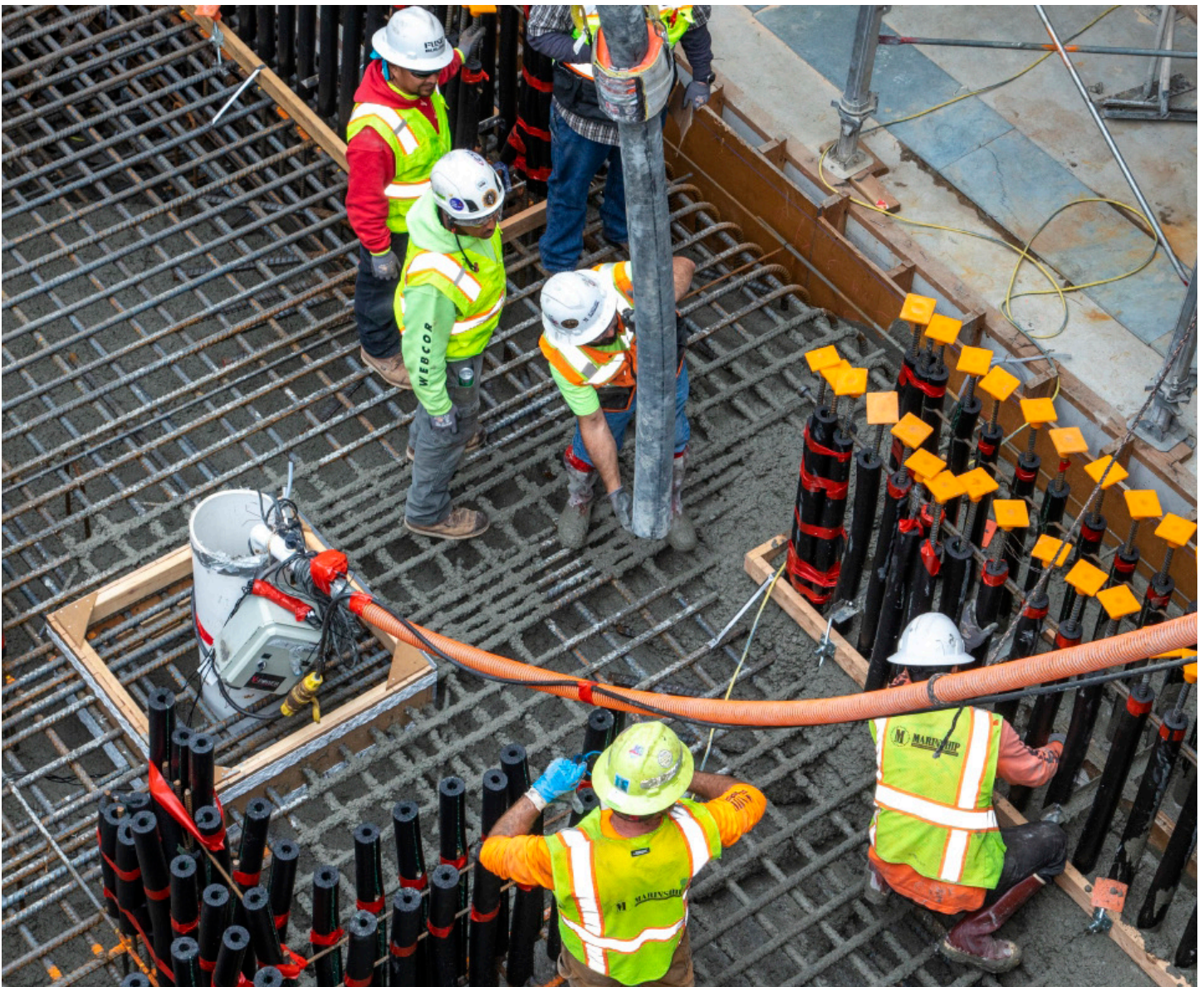
Southeast Wastewater Treatment Plant: Biosolids Digester Facilities Project: Facility 610 (Anaerobic Digestion). Reinforcing for mat slab at B615 basement.
