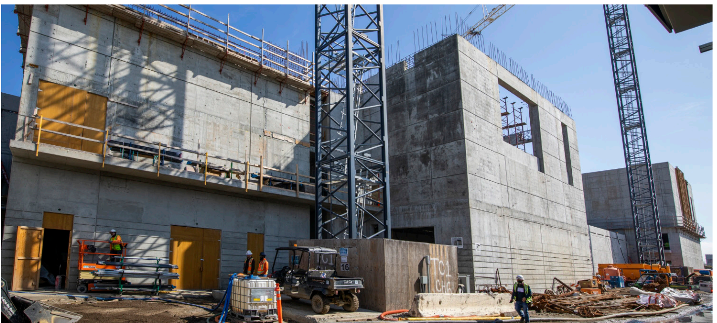
Southeast Wastewater Treatment Plant (SEP), Headworks Facility Project: Headworks Electrical Area, Screening Handling Area, Grit Tank Area, and Grit Handling Area.
