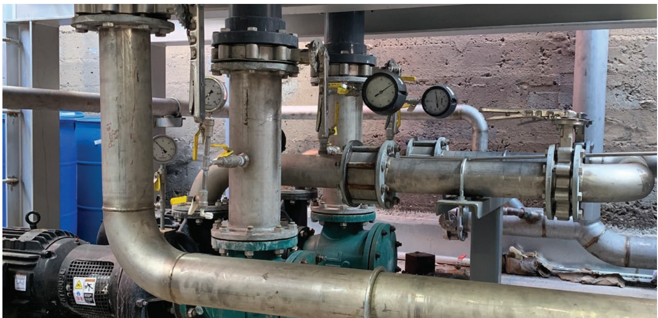
The onsite reuse system captures, treats, and reuses foundation drainage for producing steam to heat downtown buildings in San Francisco.
