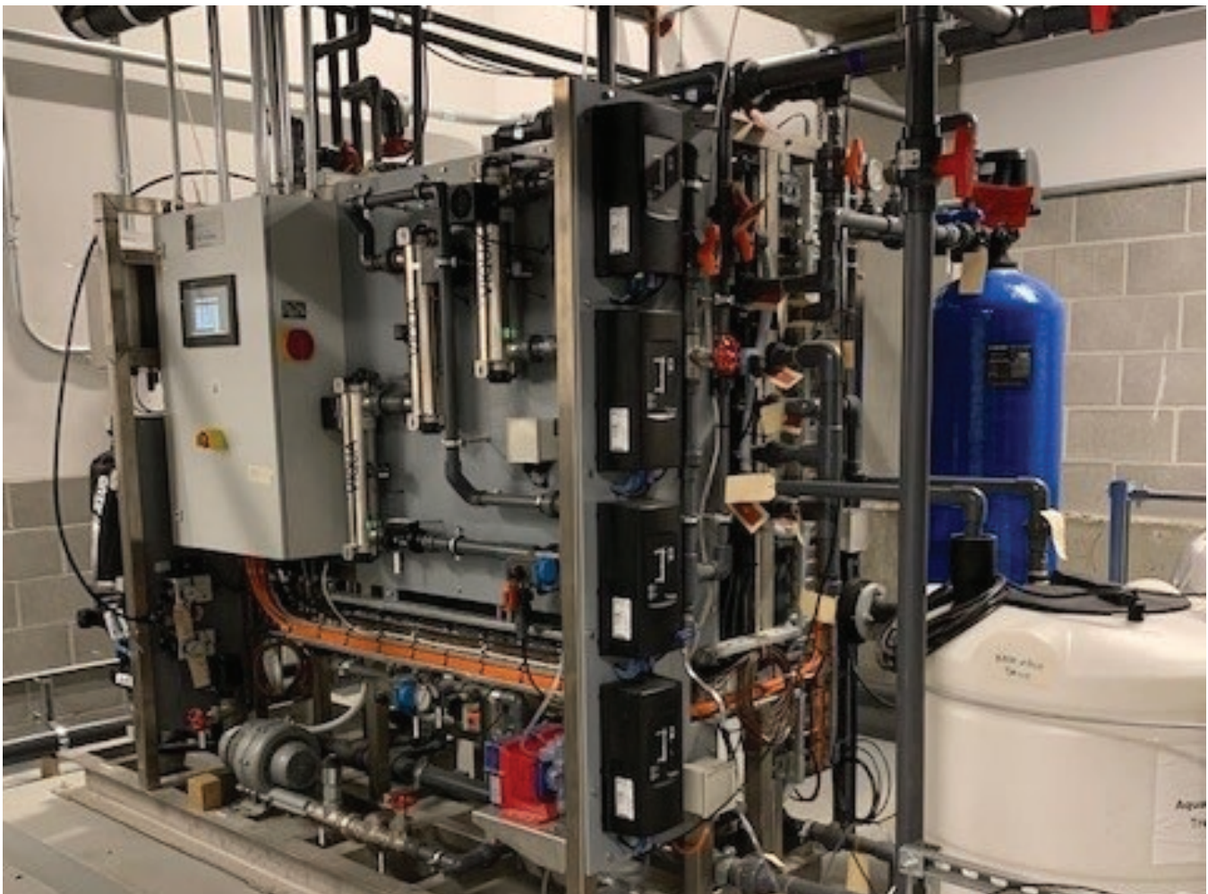
Onsite reuse system treatment skid at 49 South Van Ness (image courtesy of Aquacell)
