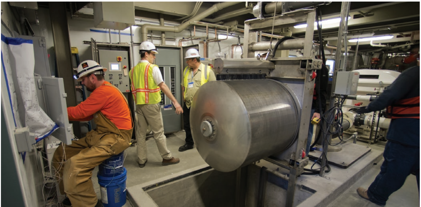
Inside the Bay heating and cooling room at the Exploratorium (image courtesy of Amy Snyder © Exploratorium, All rights reserved)
