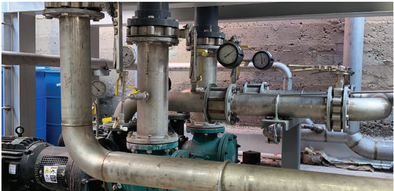
The onsite reuse system captures, treats, and reuses foundation drainage for producing steam to heat downtown buildings in San Francisco.
