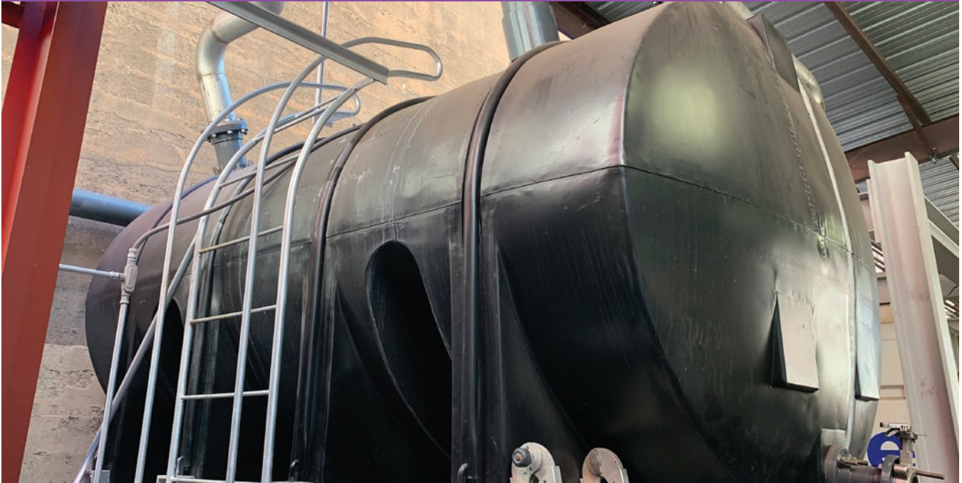
Onsite reuse system at ECSF
