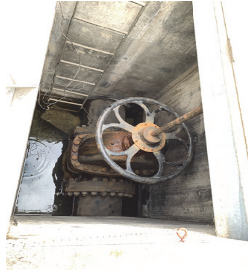
Typical Valve Requiring Installation of Additional Valve for Safe Entry
