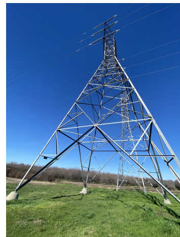
Transmission Line 7/8 Tower 508S Looking North
