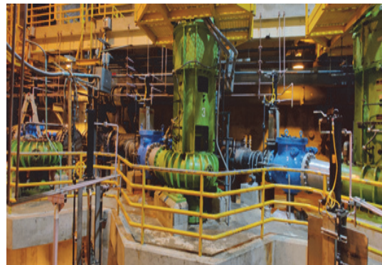
Existing Dry Weather (DW) Pump
