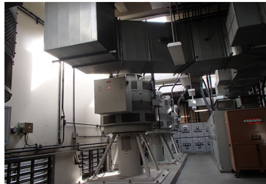
Pumps to be Replaced by Project
