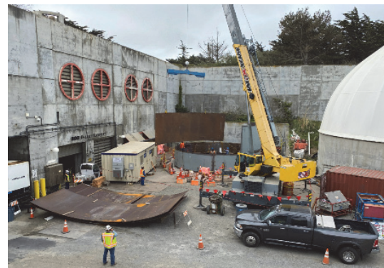
Contractor began erection of the Building 741 Digester Gas Holder tank assembly in June 2021
