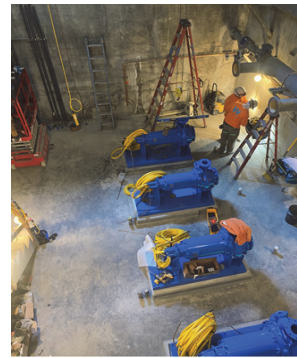
MAIN PUMPS ARE INSTALLED IN PUMP ROOM
