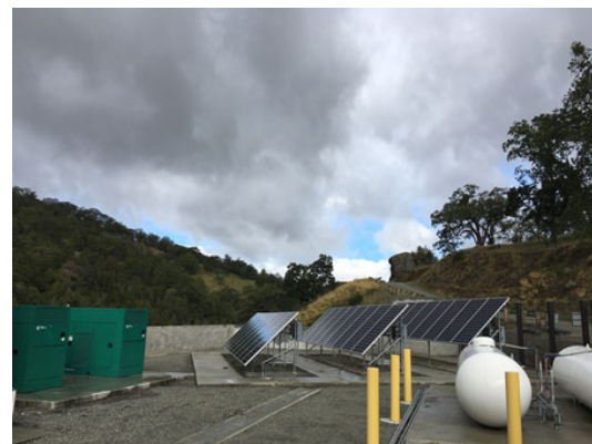
PV System, Backup Generator and Propane Tank
