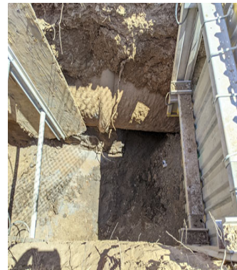
Void beneath pipeline discovered during leak investigation
