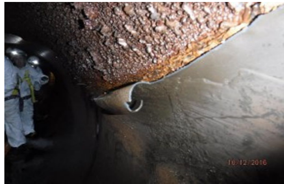
Lining Disbondment and Scaling
