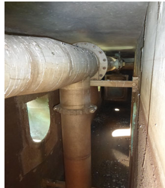
Example of air distribution piping inside a filter gullet to be used at HTWTP
