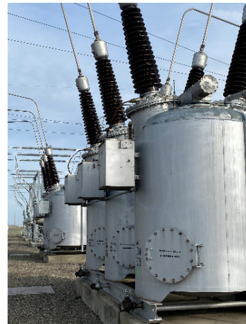
Old Oil Circuit Breakers to be Replaced
