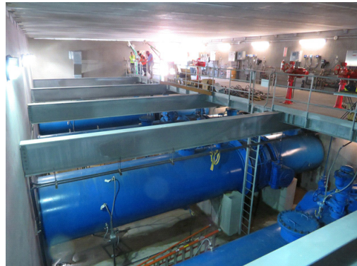
SJPL#1-4 with isolation valves within Tesla Valvehouse
