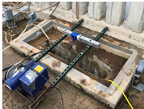
Bulkhead gate slot at top of dam and setup for underwater camera inspection
