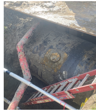
Additional pothole location showing previous repair
