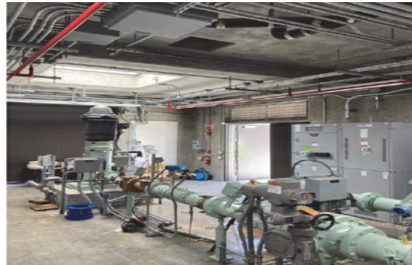
Typical well site
