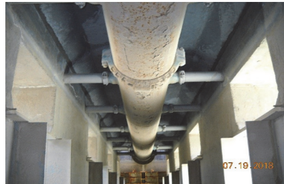
Pipe Corrosion in Air Scour Tank
