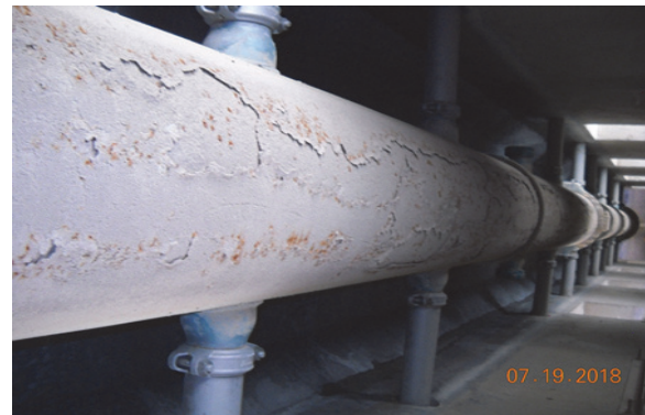
SVWTP Pipeline Corrosion
