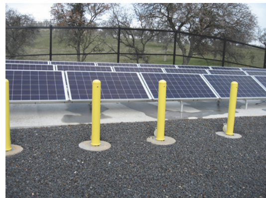
Oakdale Valve House No. 4 Solar Facilities
