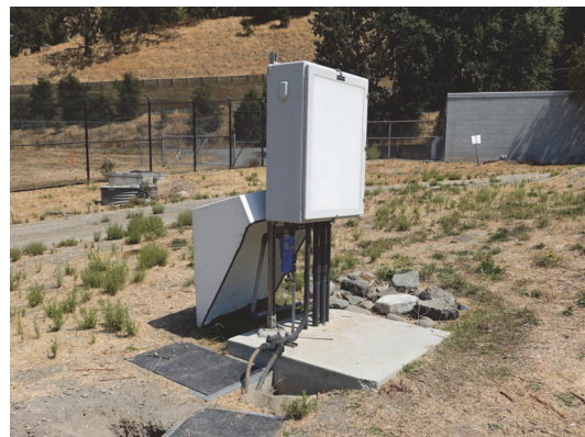
Sunshade and Pressure Relief Valve to be installed at the SABPL Chemical Analyzer Cabinet
