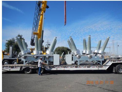
Oil Circuit Breakers
