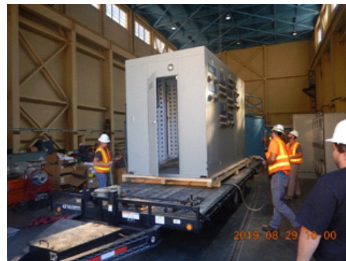
New Motor Control Board at Holm Powerhouse
