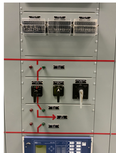
TOP: Warnerville Substation South Yard
