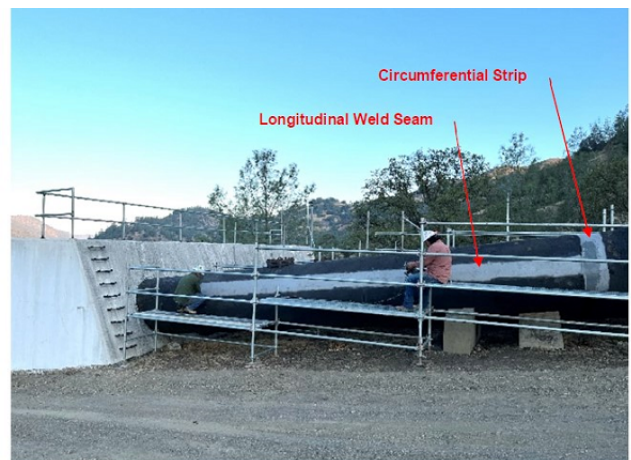
Phased Array Ultrasonic Testing inspection of a hammer forged welded steel pipe section of the penstocks
