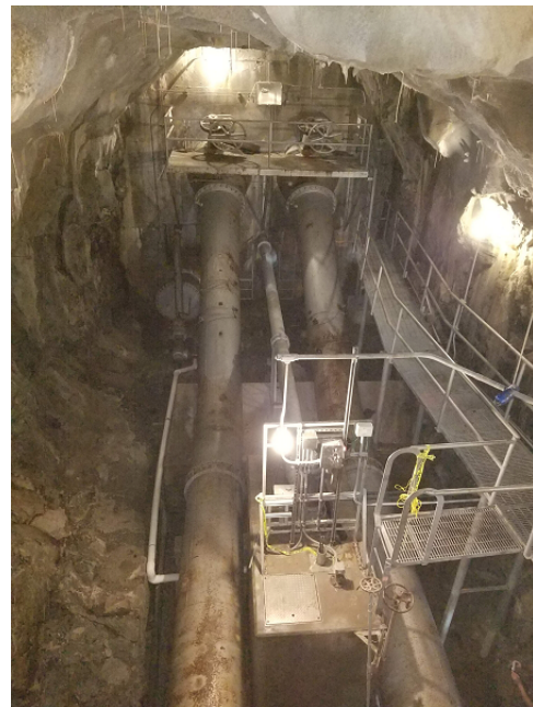
Instream Flow Release Pipe and Valves in Diversion Tunnel
