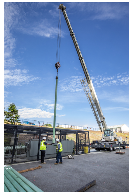
Ben Franklin Well groundwater pump pulled for inspection
