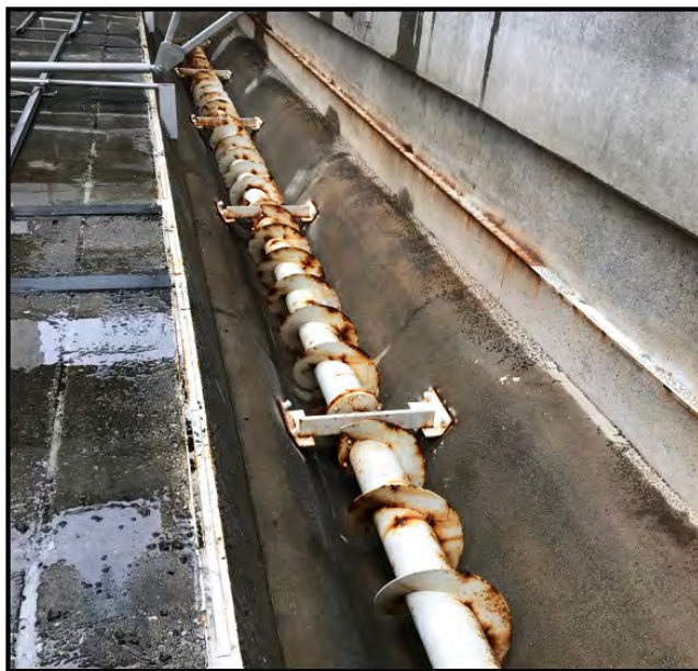
Existing Sludge Collection Auger
