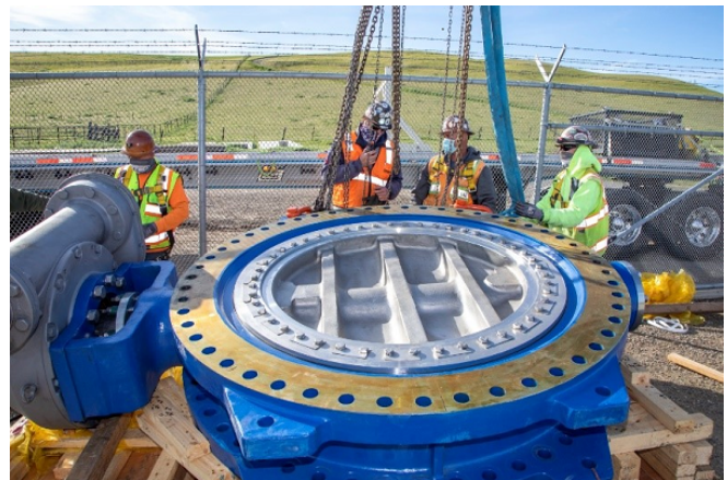
The new TUV101 prior to installation earlier this year
