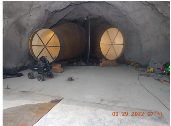
Upstream Bypass Tunnel Bifurcation Unit (This transitions the 9-foot pipe to two 6-foot pipes)
