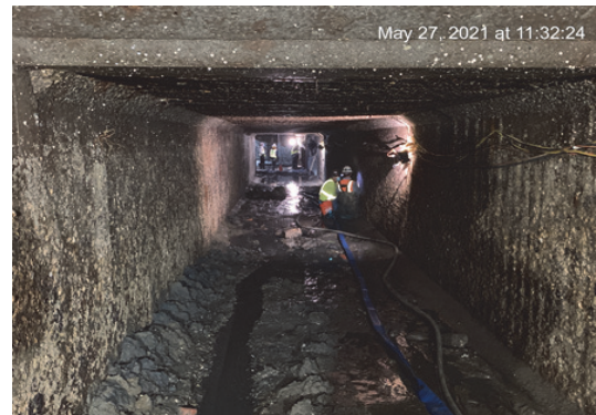
Concrete crack survey in Jackson Street CSD
