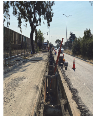
Excavation and laying HDPE flush line pipe at Cargo and Mandel St
