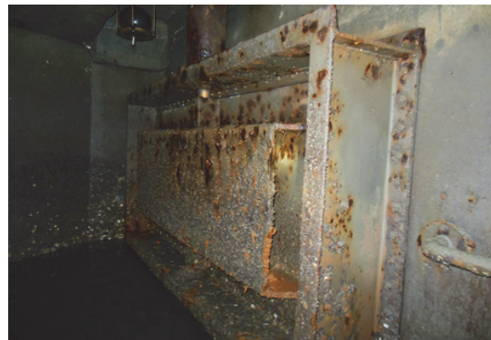
Non-operational butterfly valve at Brannan CSD
