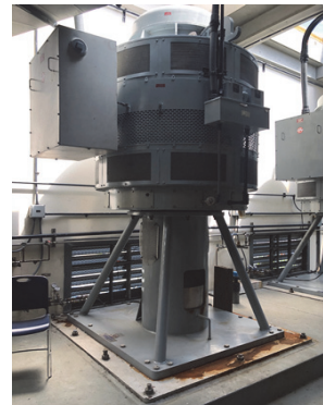
Main Pump Being Evaluated
