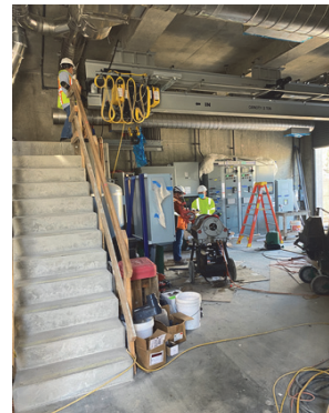
Electrical Equipment Contractor inhouse check
