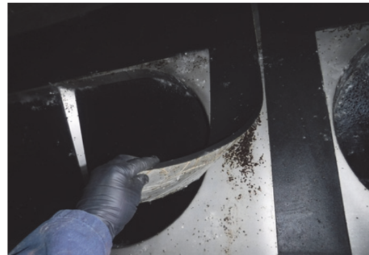
Baker St. CSD damaged backflow preventer valve
