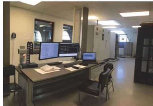
Updated Bruce Flynn Pump Station Control Room
