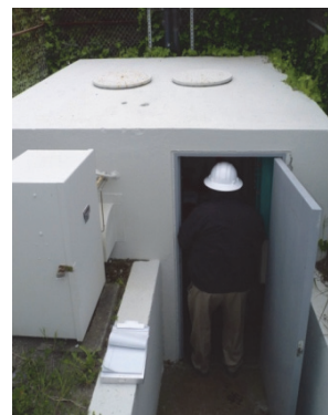
Seacliff Pump Station No.1
