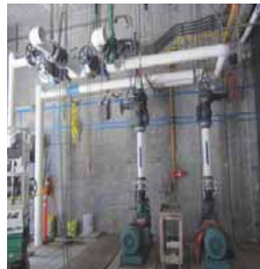
Within OSP Building 820, the Contractor installed the boiler hot water loop pump system equipment and mock-up piping in August 2020.
