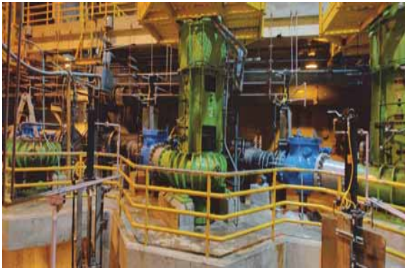
Existing Dry Weather (DW) Pump
