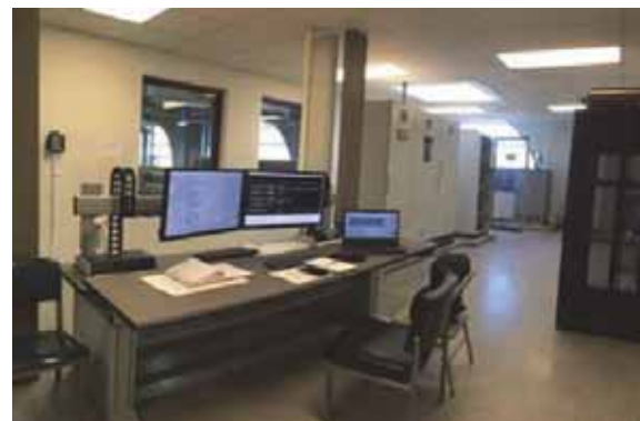
Updated Bruce Flynn Pump Station Control Room
