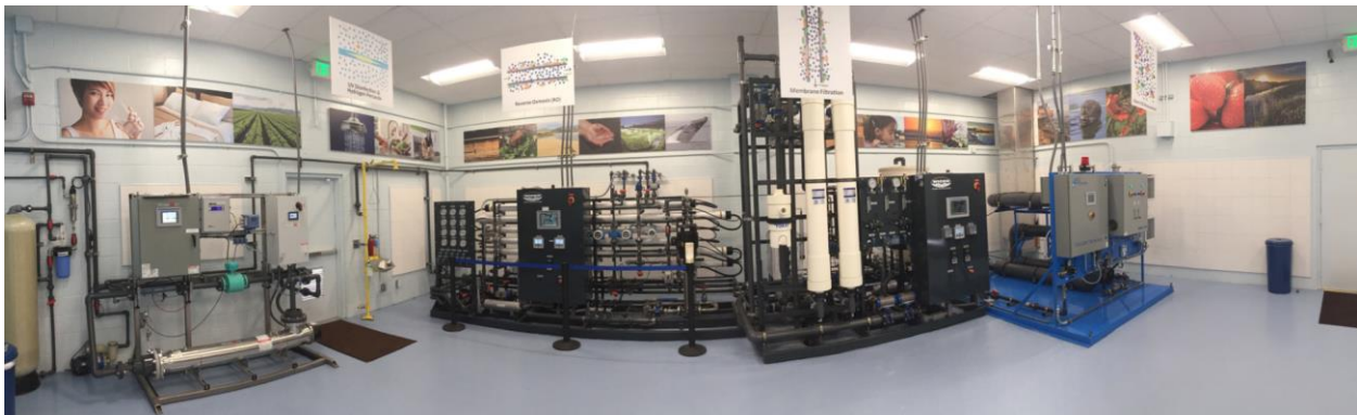
Figure 4-2: M1W Demonstration Facility
