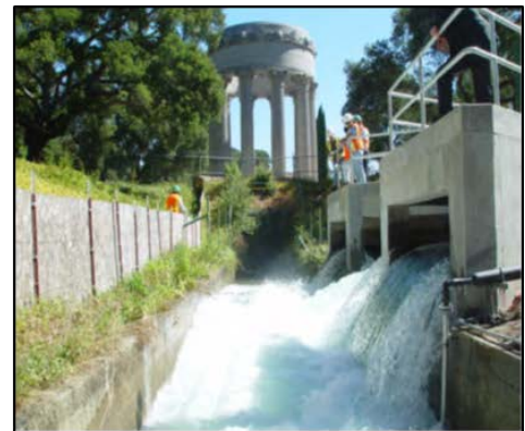
Above: Flows from the Puglas Dechloramination Facility enter the Puglas Discharge Channel for release to Upper CSR.
