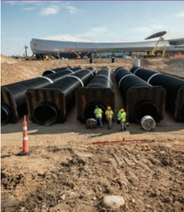
Installation of underground rainwater storage tank outside of stadium (Image courtesy of the City of St. Paul)
