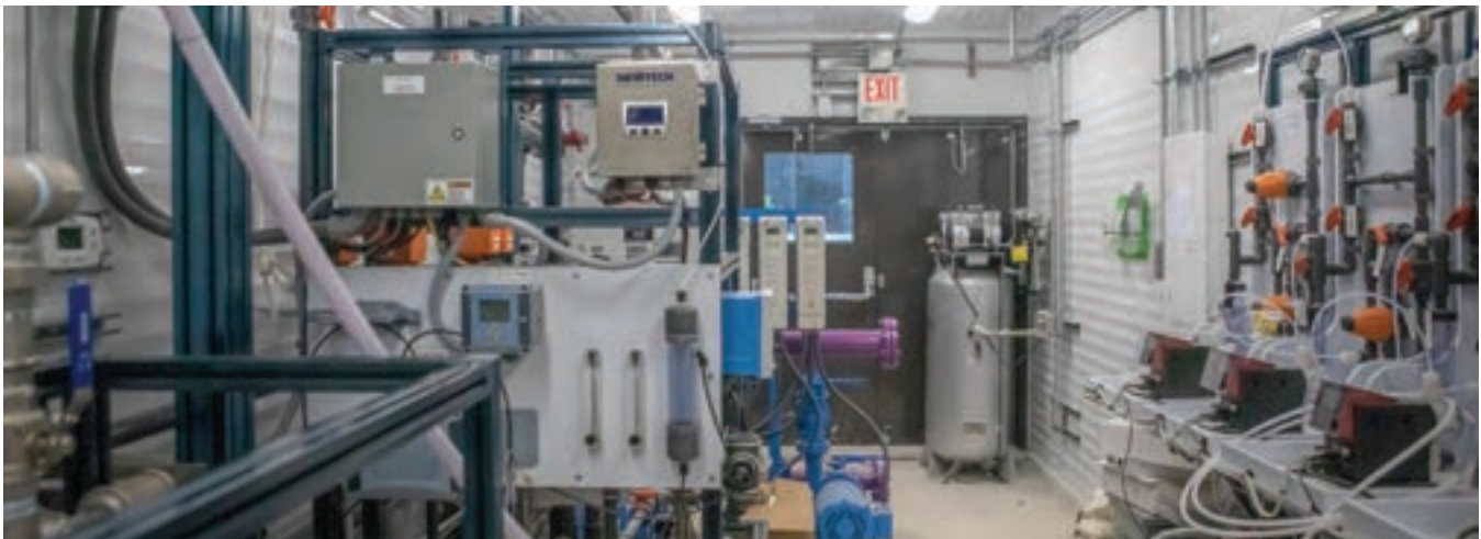
Onsite reuse system treatment room (image courtesy of Austin Water)
