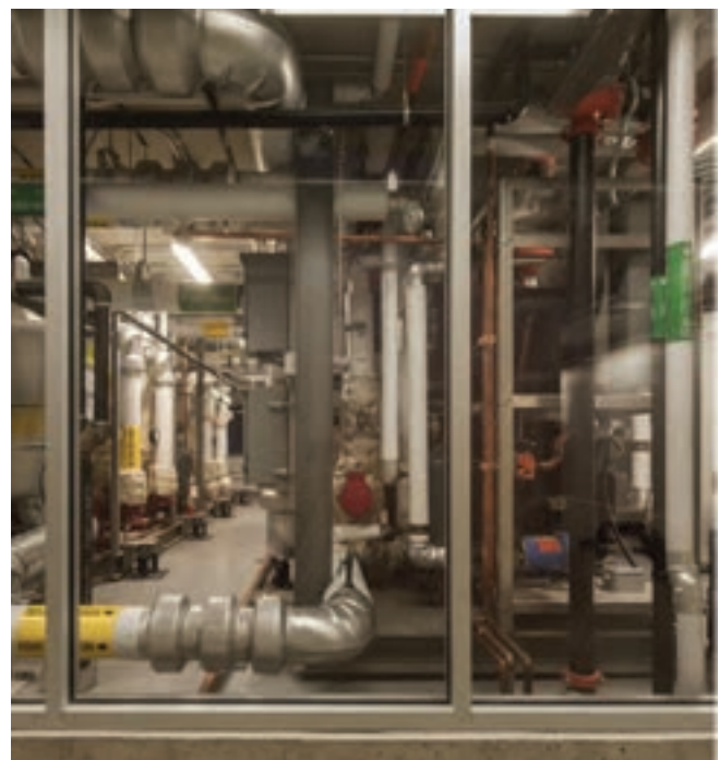
Onsite reuse system (image from Gray & Osborne Inc., Consulting Engineer's Bullitt Center Water Treatment System Engineering Report)
