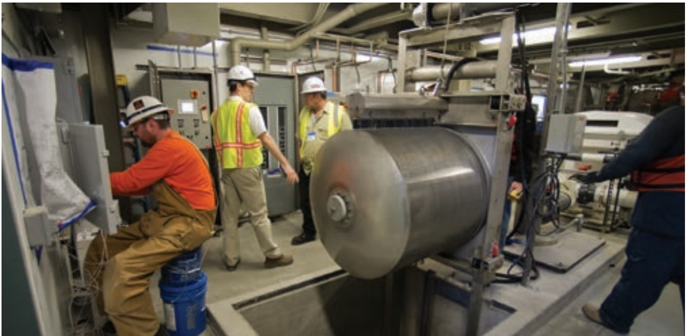
Inside the Bay heating and cooling room at the Exploratorium (image courtesy of Amy Snyder © Exploratorium, All rights reserved)
