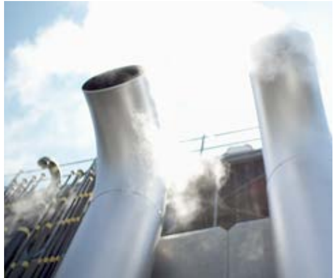
UConn Water Reclamation
