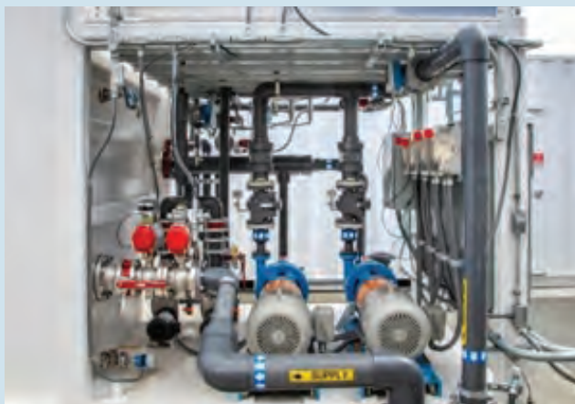
Anchor Brewing Company's Brewery Process Water Reuse System in San Francisco, CA
