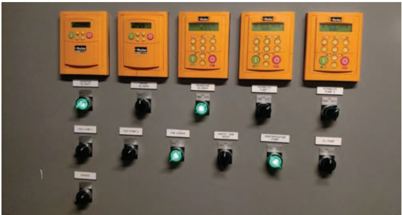
The onsite reuse system’s control panel (image courtesy of NSU)
