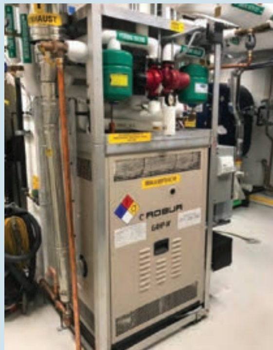
Wastewater Heat Recovery System at the Solaire in New York City (image courtesy of Natural Systems Utilities)
