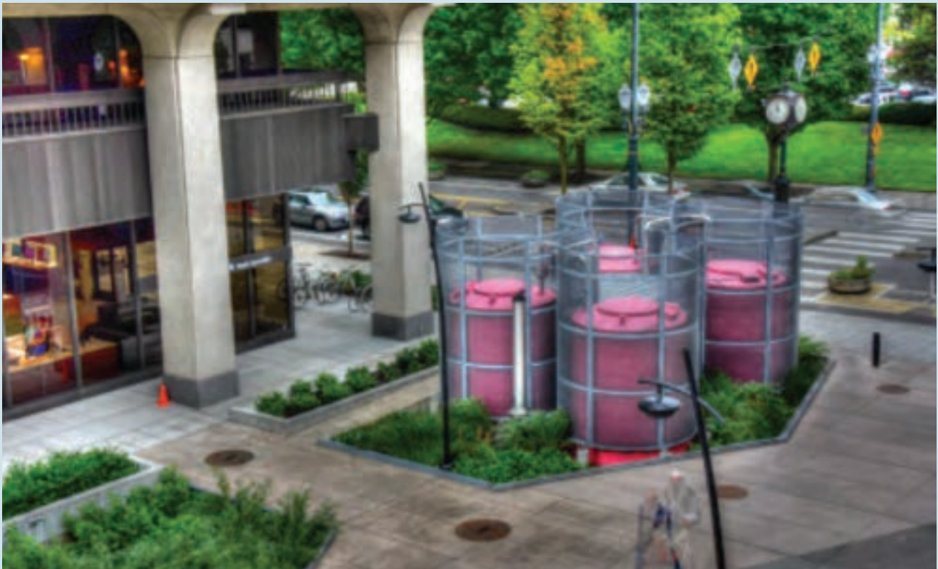
Hassalo on Eighth Wastewater Treatment System (image courtesy of Jim G. Maloney/Biohabitats, Inc.)
