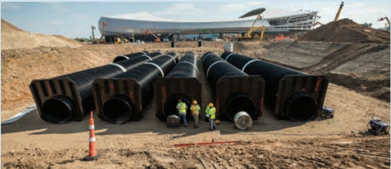
Installation of Underground Rainwater Storage Tank at Allianz Field in St. Paul, MN (image courtesy of City of St. Paul)
