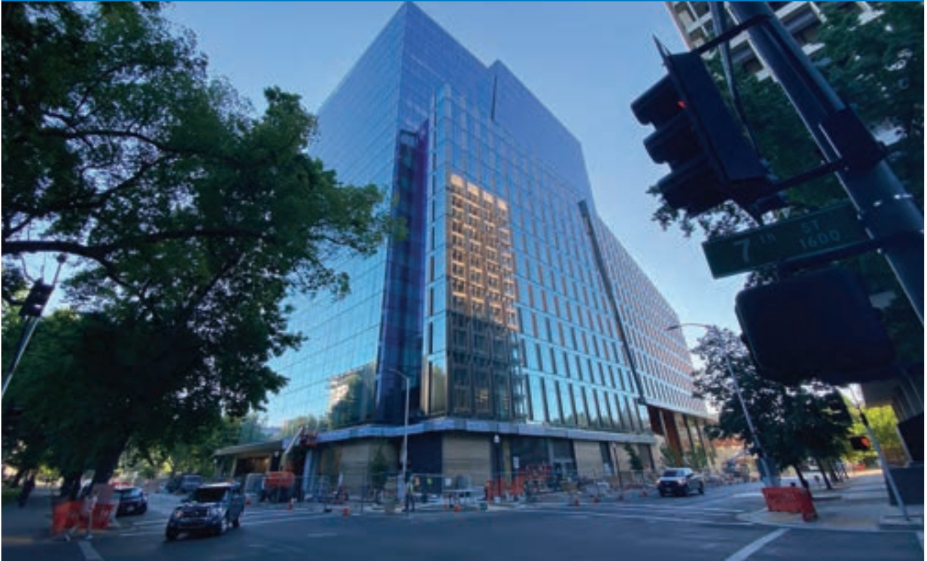
DGS Natural Resources Building under final stage of construction (image courtesy of HTEC)
