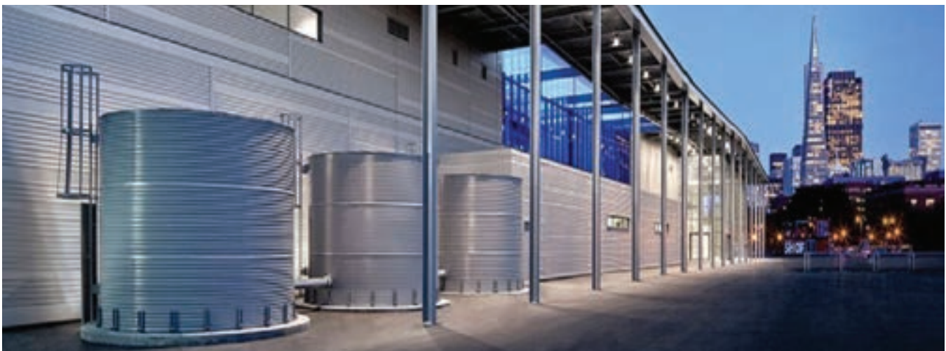
The rainwater cisterns at Pier 27 (image courtesy of San Francisco Public Works)
