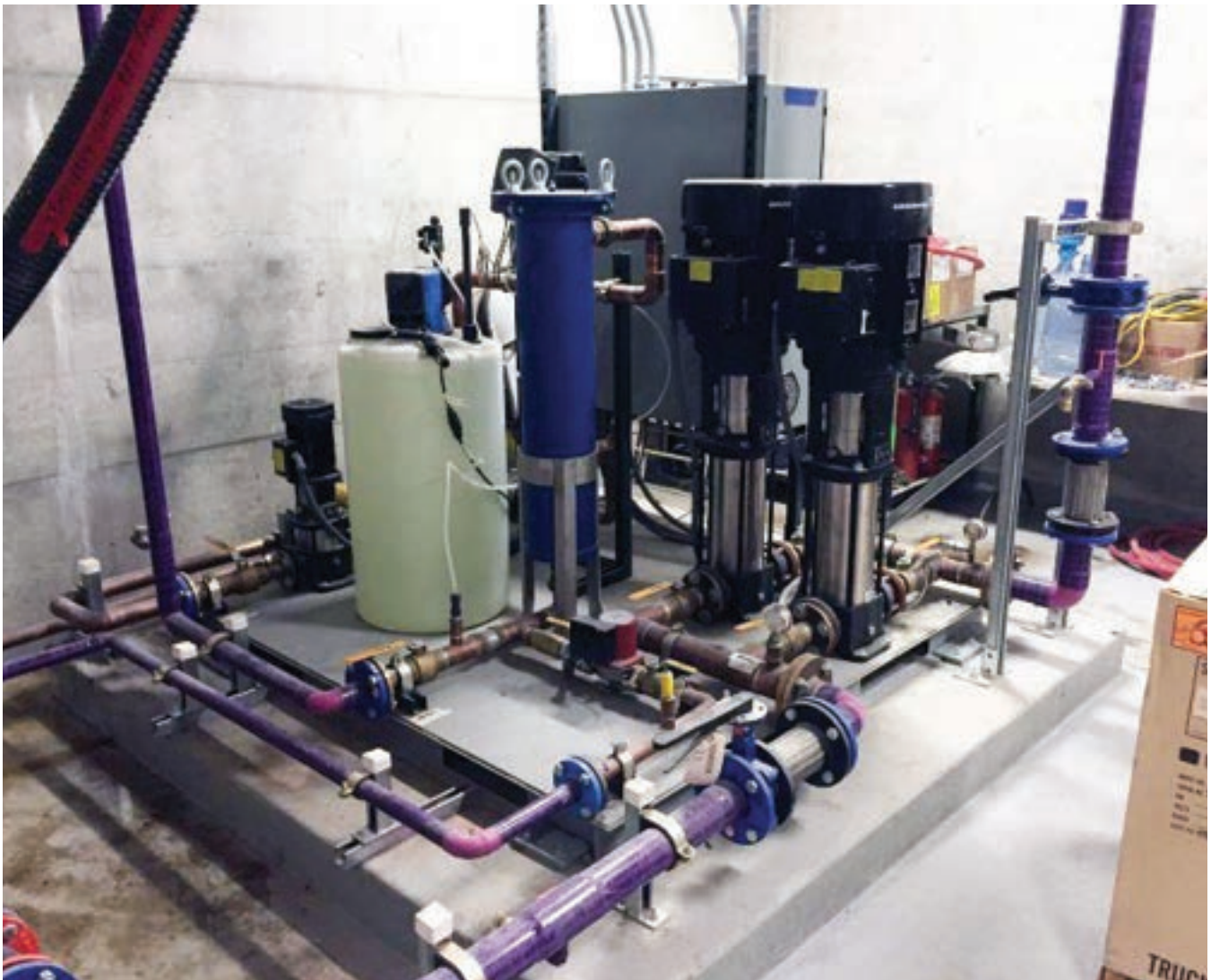
The San Francisco Museum of Modern Art's onsite water system (image courtesy of Bob Reuter)
