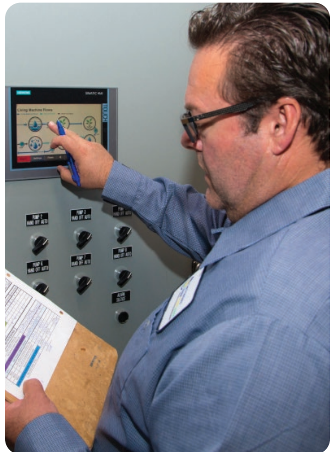
The Treatment System Manager can train building staff to perform routine inspections and maintenance.
