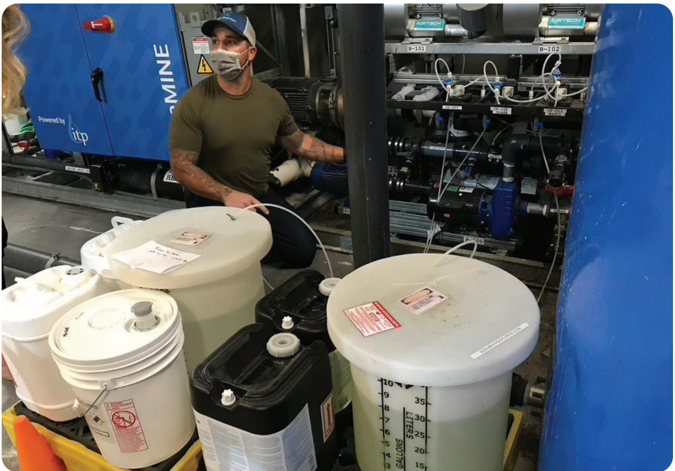
The Treatment System Manager of the combined graywater and rainwater treatment system at 1550 Mission uses chlorine to maintain a disinfectant residual to provide protection against opportunistic pathogens such as Legionella.
