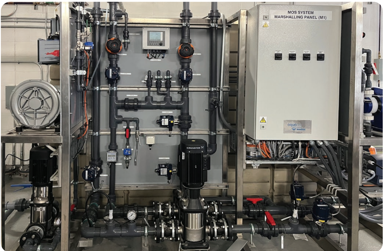
Mission Rock's district-scale blackwater treatment system is the first of its kind in San Francisco. The system will meet all of the demands for toilet and urinal flushing and irrigation and is estimated to offset about 55% of the development's total water demand.
