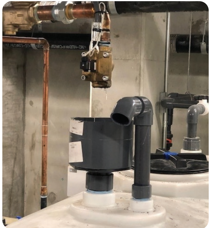
Potable make-up water is supplied to the treated water storage tank via an air gap.
