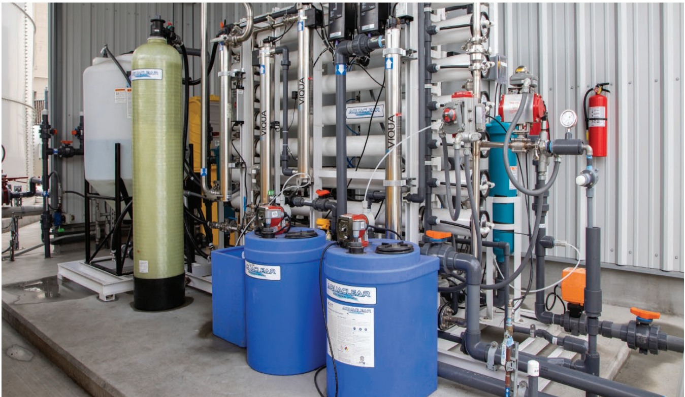
Anchor Brewing Company's brewery process water recycling system
