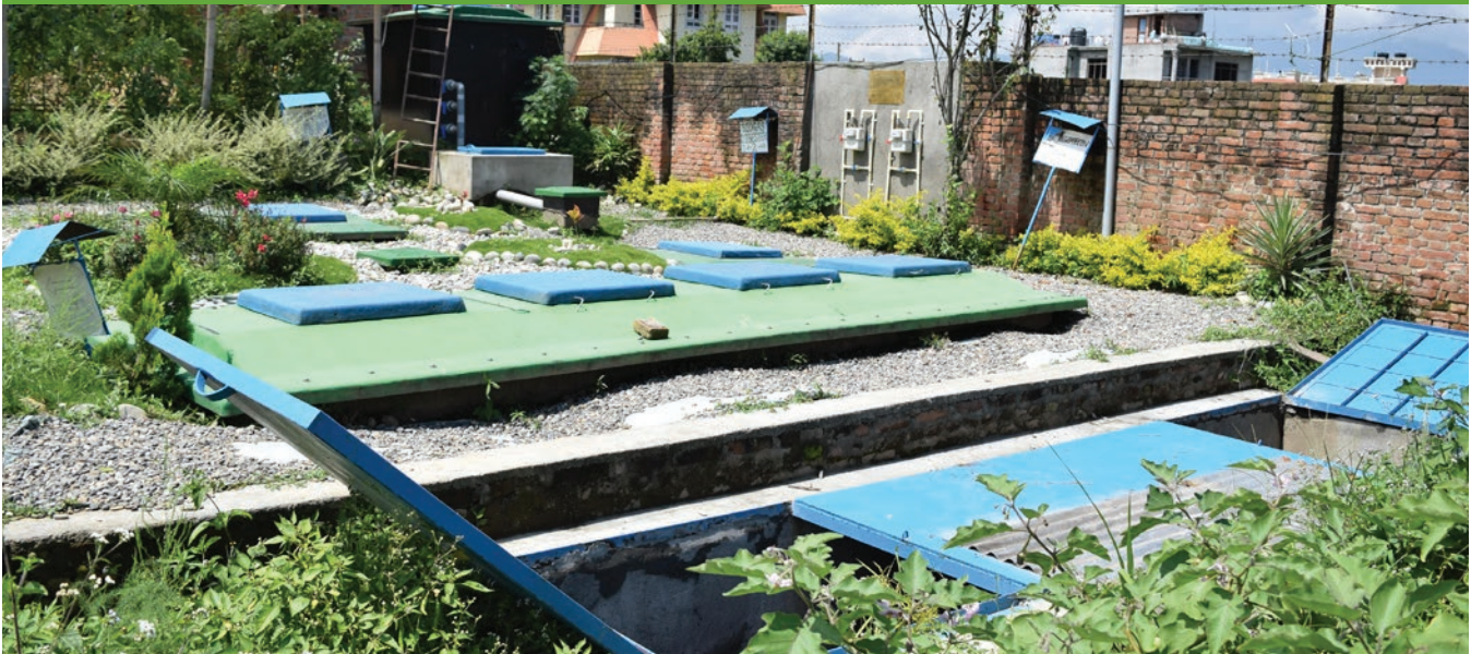
A view of the treatment plant's prefabricated modules (photo courtesy of ENPHO)
