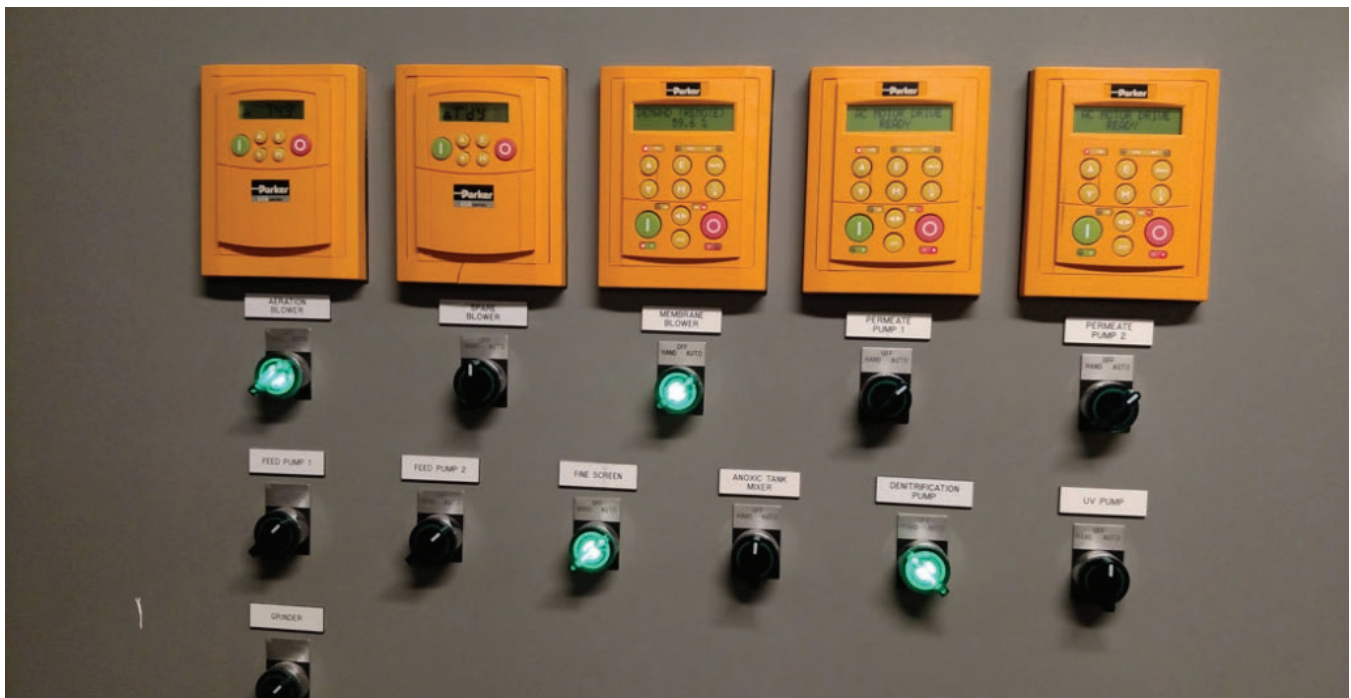
The onsite reuse system’s control panel (image courtesy of NSU)
