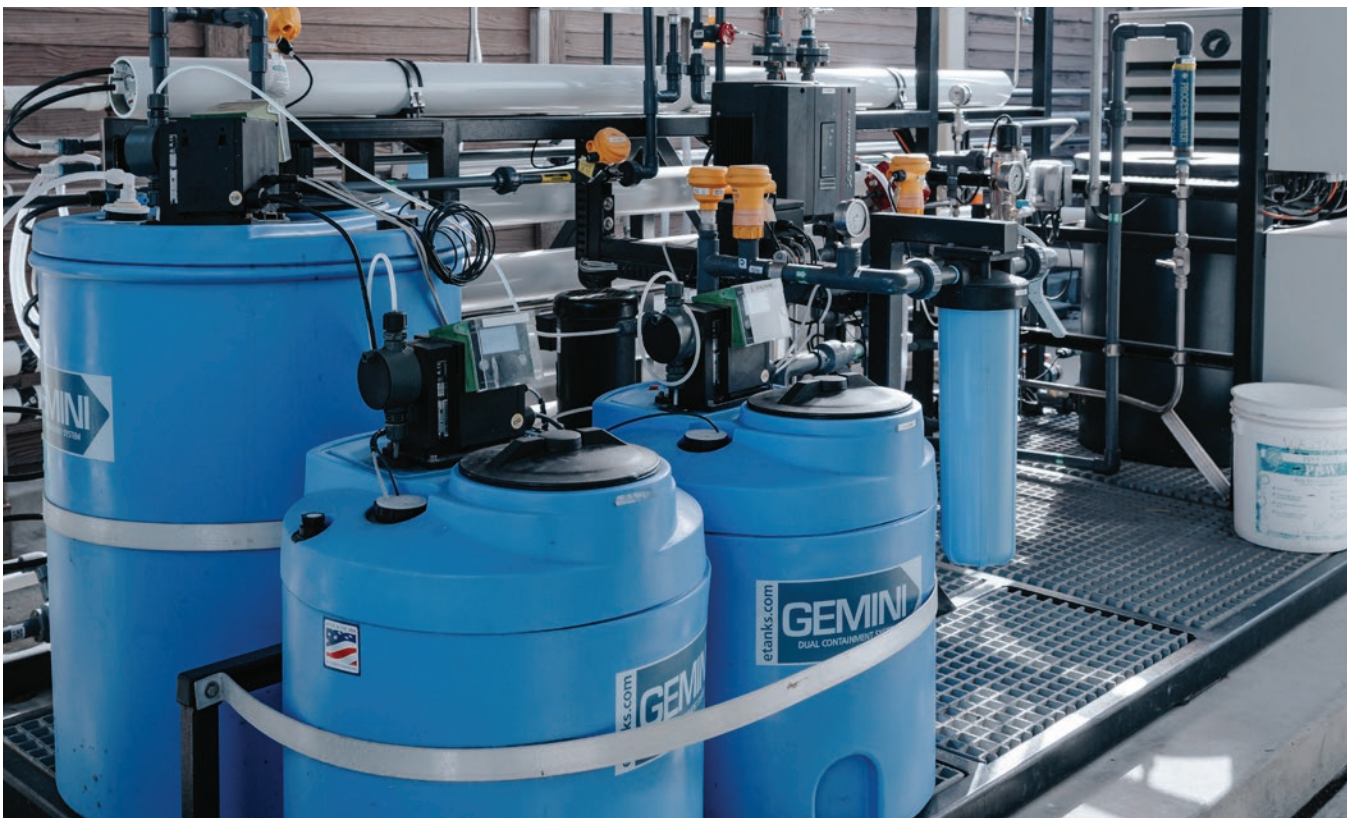
Treatment system RO skid (image courtesy of Seismic Brewing)
