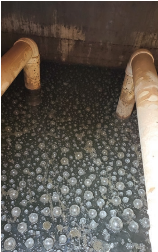
Tarabo anaerobic treatment at work (image courtesy of Water 1st)
