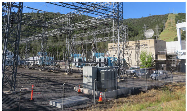
Existing Moccasin Switchyard
