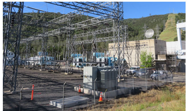
Existing Moccasin Switchyard
